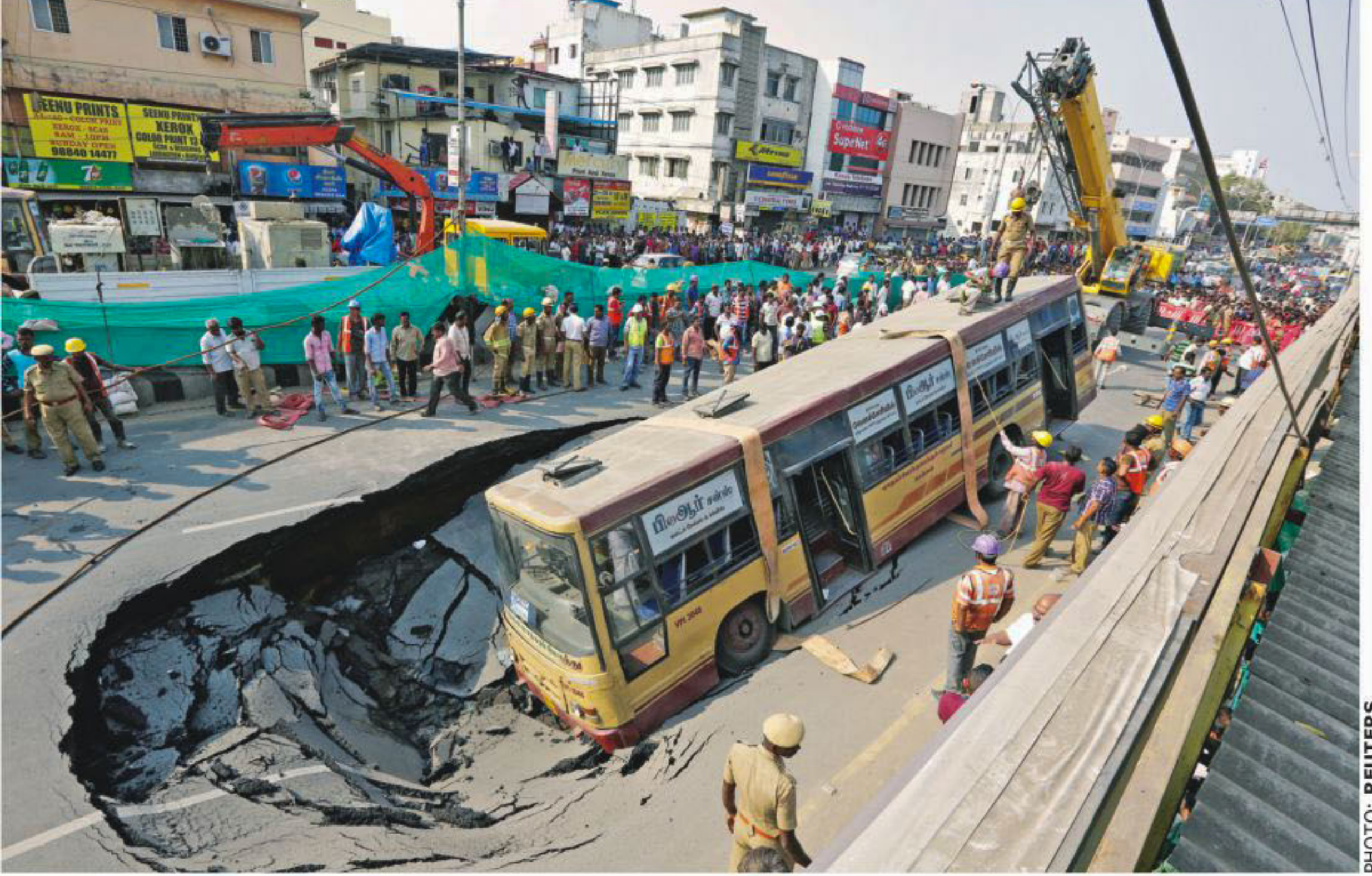
Rescue workers prepare to lift a passenger bus from a pit after a road caved in, in Chennai, India, yesterday. According to Chennai Metro Rail Limited sources, the incident happened due to the impact of a tunnel boring machine which was drilling beneath the road, a few metres beside the spot where the road caved in. No one was injured.
