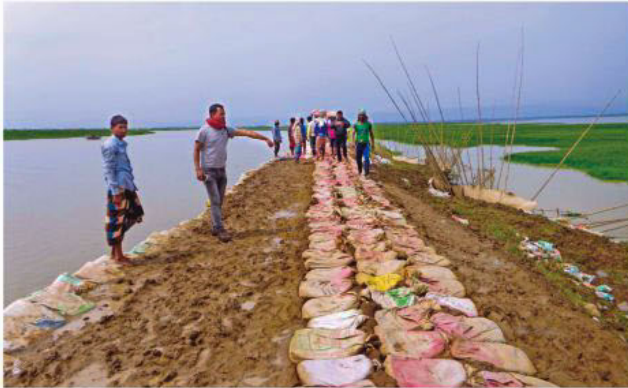
Villagers take matter into their hands after waiting for months for the authorities concerned to repair the three-kilometre damaged portion of an embankment in Sunamganj. The photo was taken from the Bagiani village portion of the levee recently.
