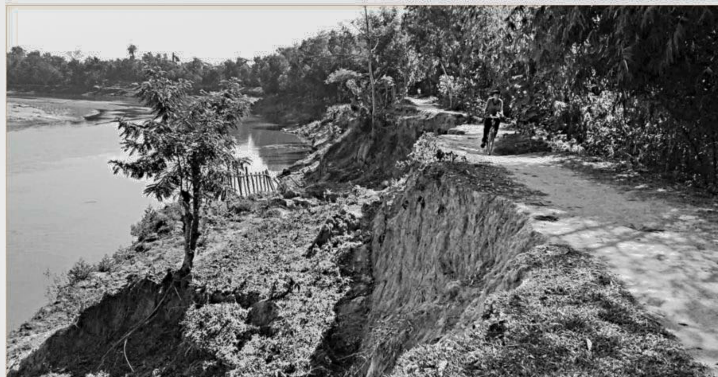
A portion of flood control embankment collapsed at Mondira village in Kulaura upazila of Moulvibazar as the Monu river started swelling.
