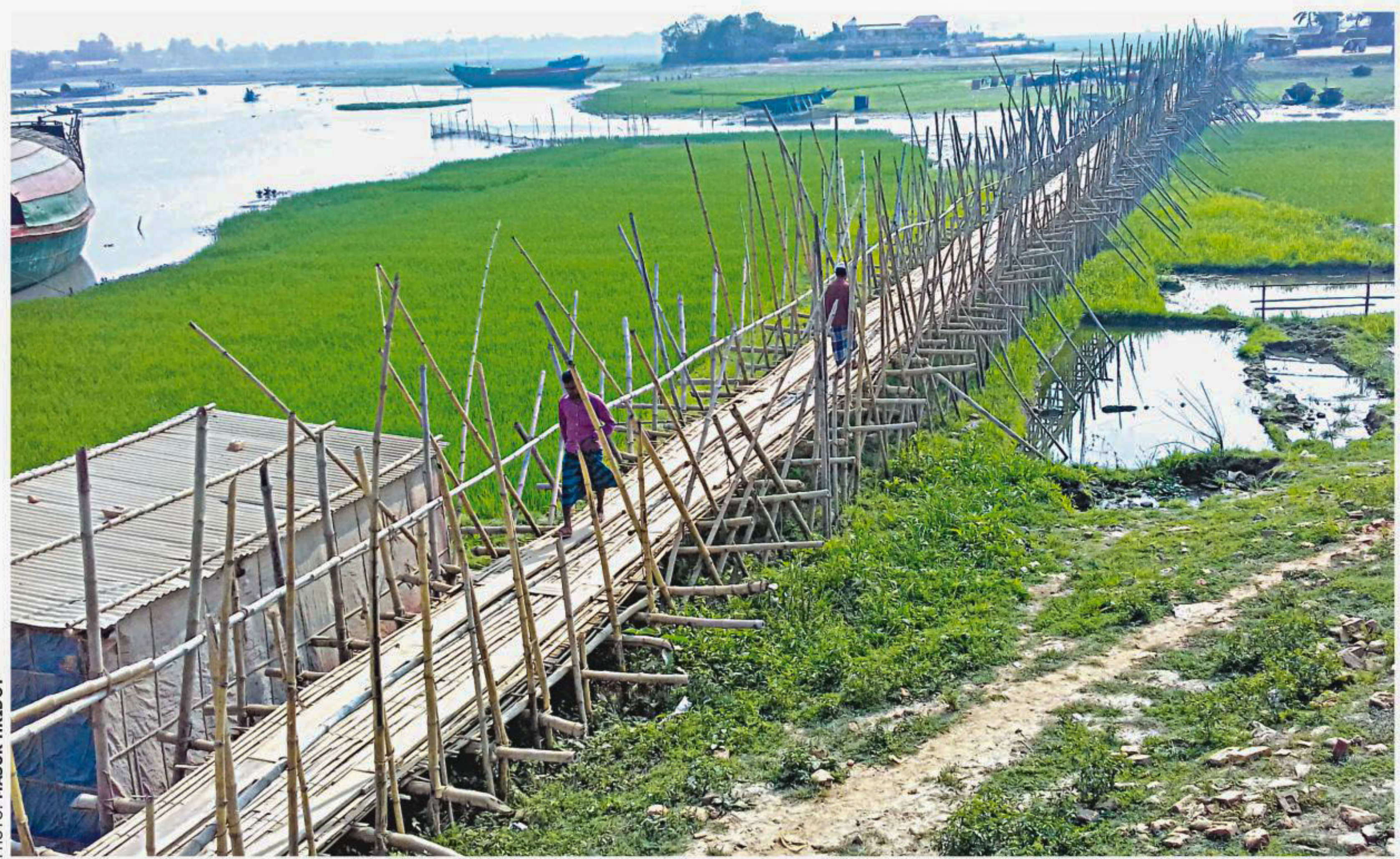
Thousands of people use this 20-year-old rickety bamboo bridge over the Chhetra river in Brahmanbaria's Sarail upazila. People of two unions cross the 1,000-foot bridge on foot and on bicycles and bikes. They have been demanding a concrete bridge there for long but the authorities have not taken any steps yet.
