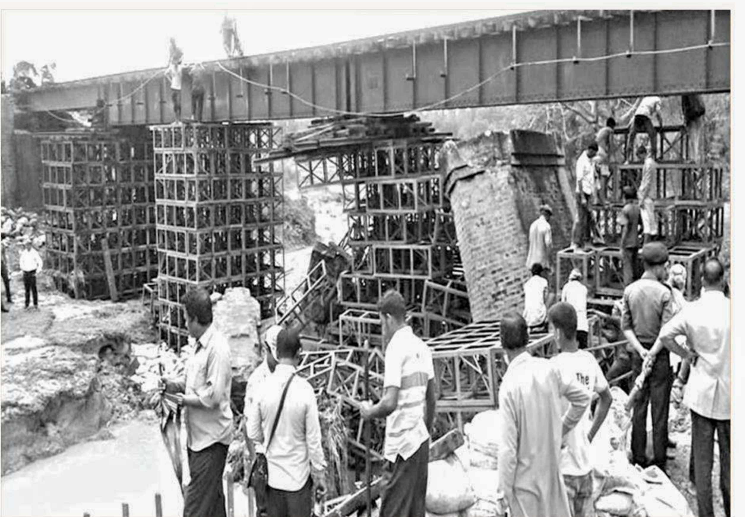
Workers yesterday repair a railway bridge which collapsed due to heavy rain in Madhabpur upazila of Habiganj on March 30.
