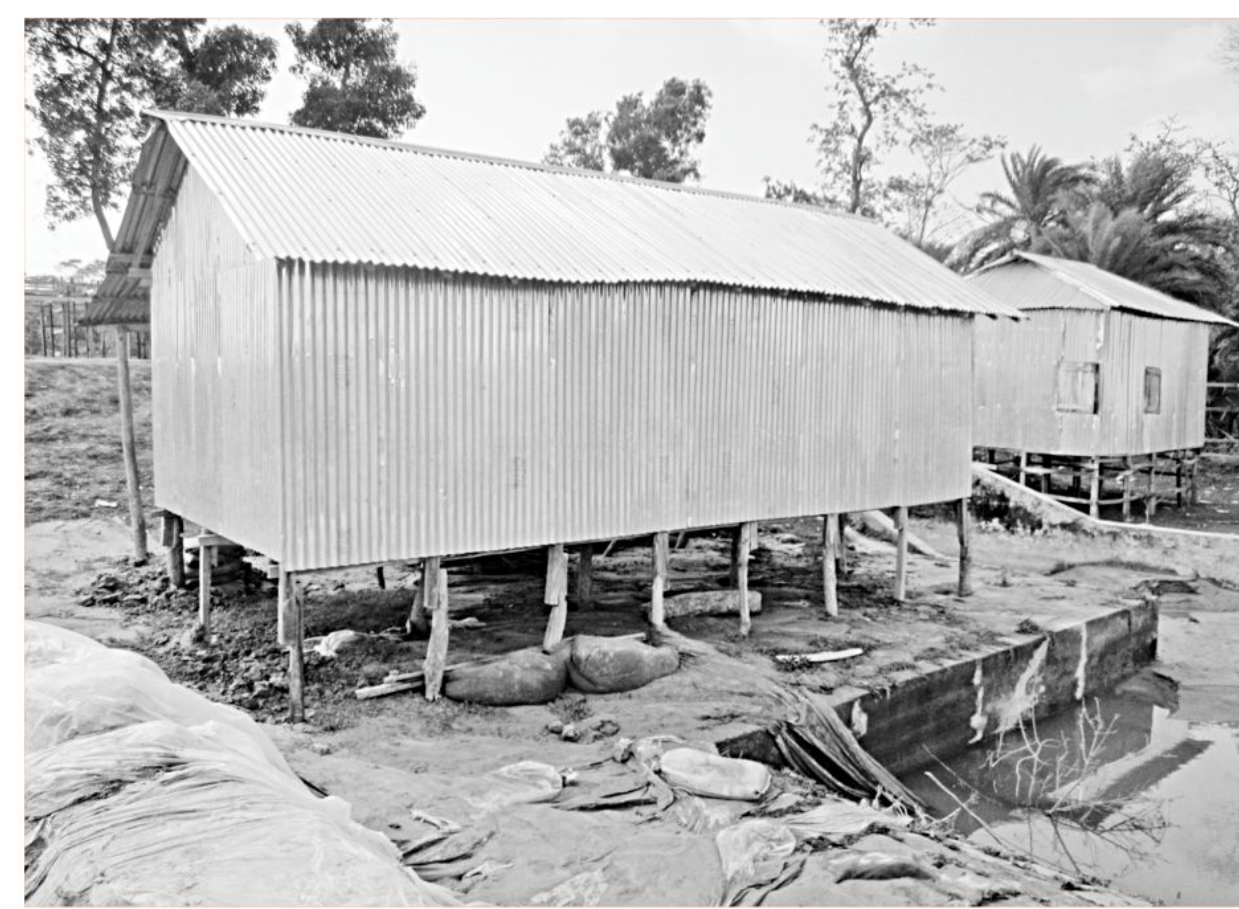
Under-construction wooden structures on both sides of a sluice gate of WDB near Payra port in Kalapara upazila of Patuakhali.
