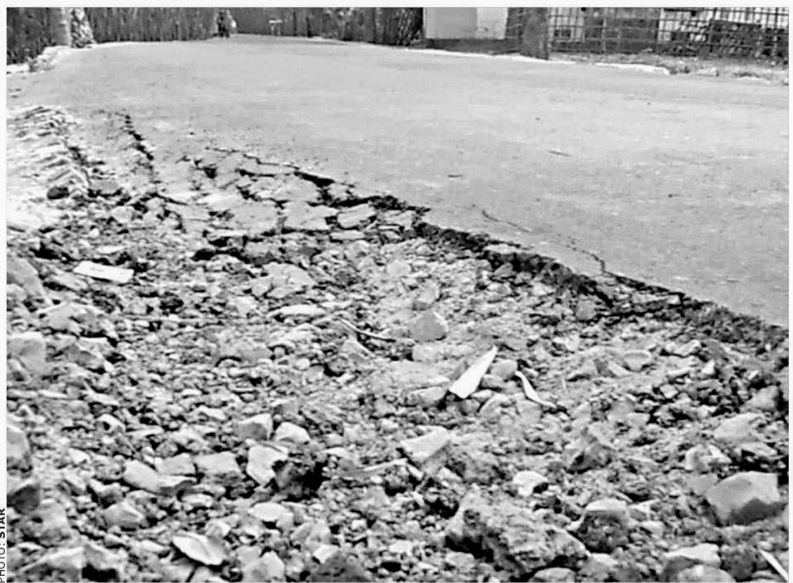
Mahendranagar-Mostafi road, being reconstructed under Local Government Engineering Department, has broken down in Mahendranagar area of Lalmonirhat Sadar upazila due to 'low quality' materials used in the repair work. PHOTO: STAR
