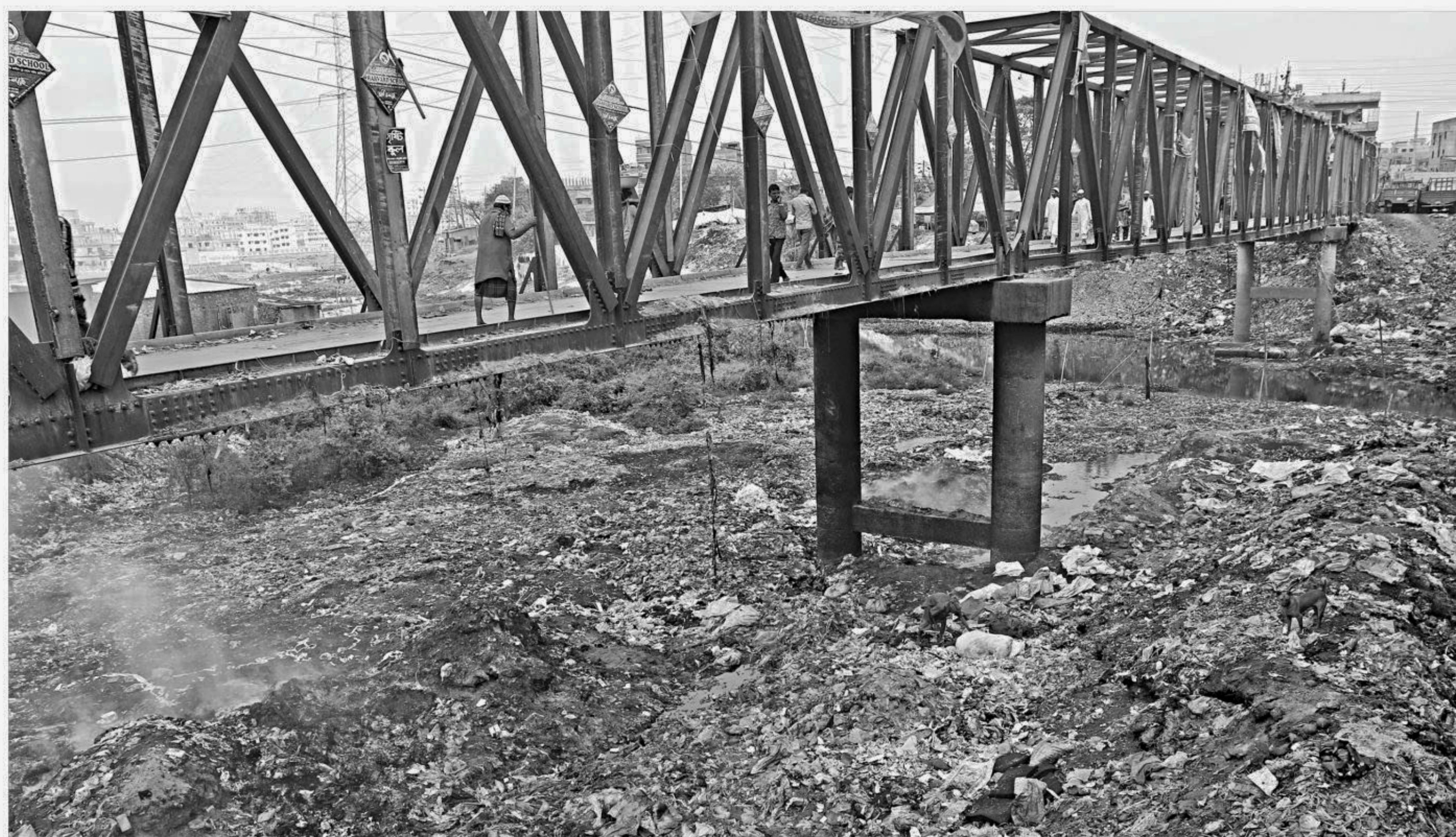
Garbage is dumped in piles under the Lohar Bridge in Kamrangirchar area of Dhaka and set alight every day, harming the environment. Not just authorities concerned, a collective effort of all is needed to prevent this mindless act. The photo was taken recently.
