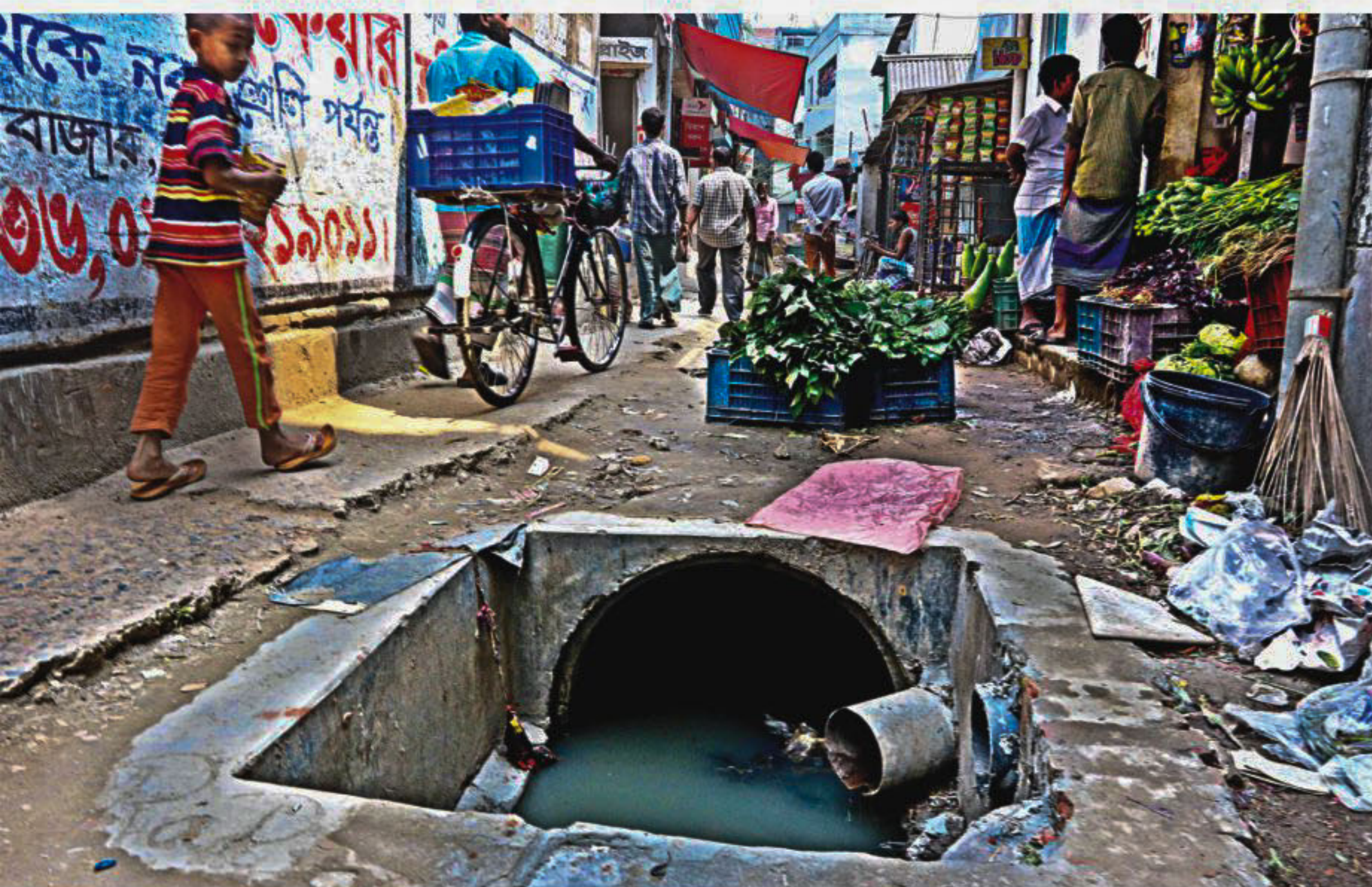
A child walks by an open sewerage pit in Peyarabagh area of Moghbazar under Ward 35 of Dhaka North City Corporation. Unsafe practices go unabated in the country although the High Court only a few days ago directed police to sue six government employees and a contractor for negligence and violation of public safety after a man, Shanu Miah, died falling into an uncovered box culvert in the capital's Paltan area on March 6. The photo was taken on Tuesday.
