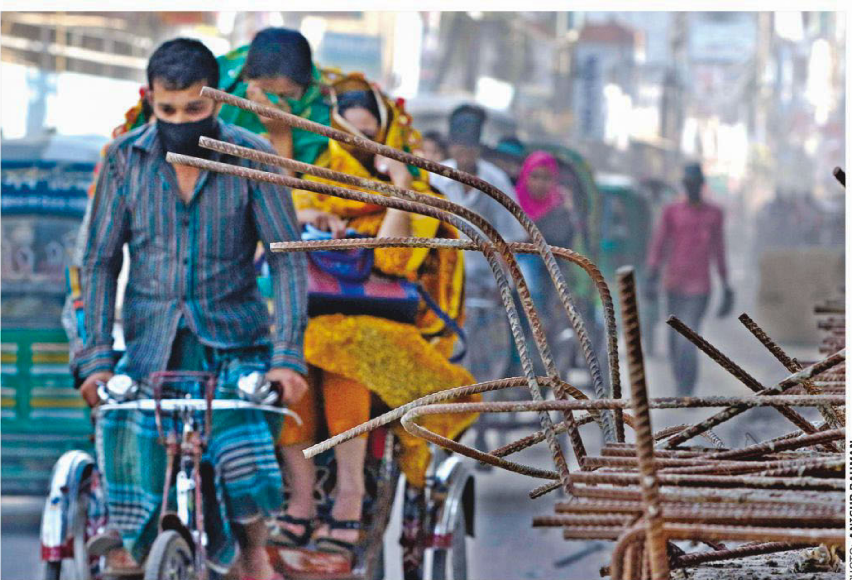
Iron rods stick out to oncoming traffic from a girder of the under-construction Moghbazar-Malibagh flyover near the city's Malibagh level crossing yesterday. The contractor has been building the structure for several years which already led to some serious accidents. Only a day ago a girder fell from a pillar of the flyover at this location, killing one and injuring two others.
