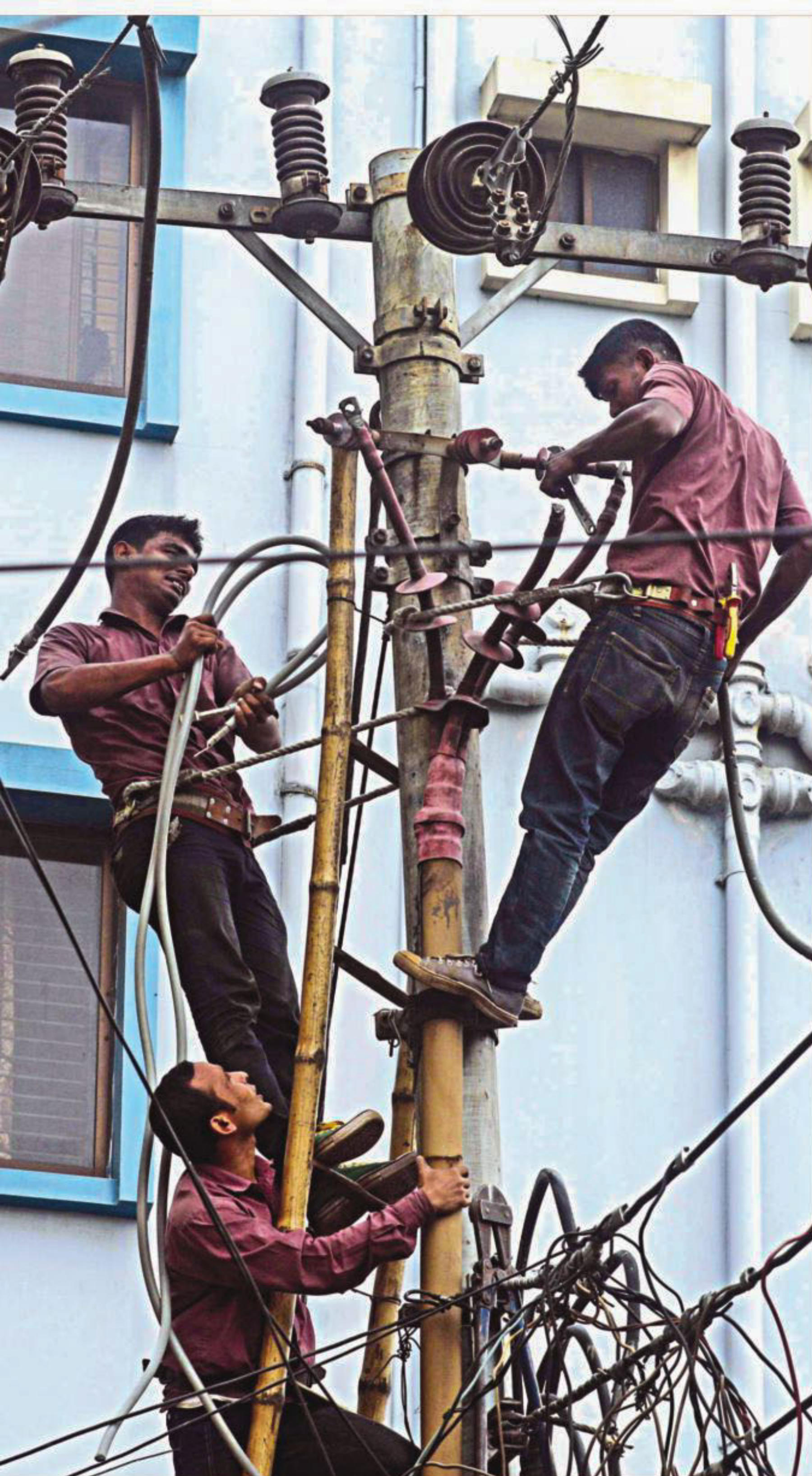
Without any proper safety measures, workers of Dhaka Power Distribution Company Limited work on a roadside electric pole in the capital's Tejgaon area. Workers involved in high-risk jobs often fall victim to fatal accidents for a lack of protective equipment. The photo was taken on Saturday. PHOTO: PRABIR DAS
