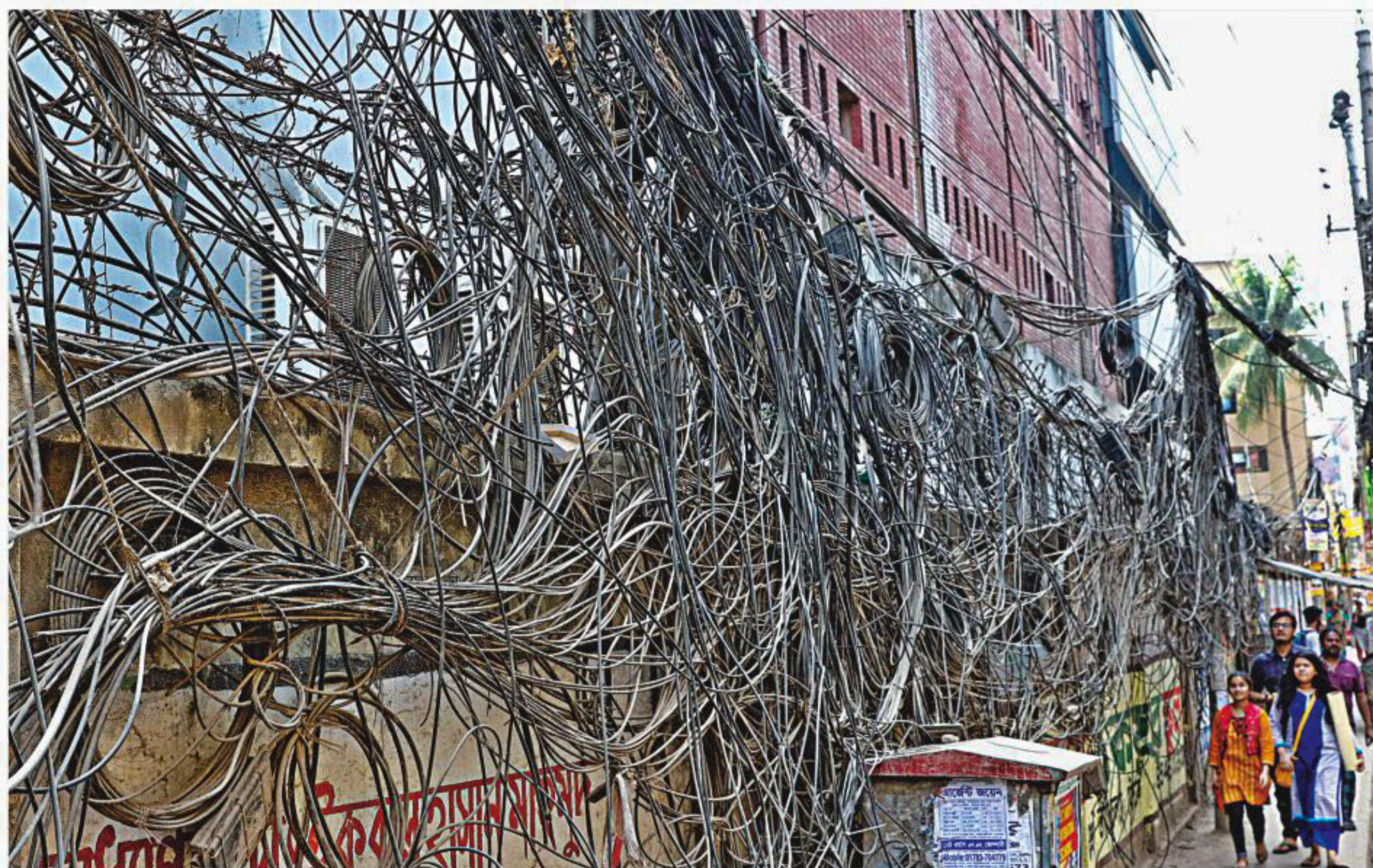
CABLE CHAOS... TV, telephone and internet cables strung haphazardly on a wall of Bangladesh Telecommunications Company Ltd's office in the capital's Moghbazar. Local internet resellers string their cables on power and telephone poles although it is against the law. Authorities remove the cables from time to time but they reappear soon.
