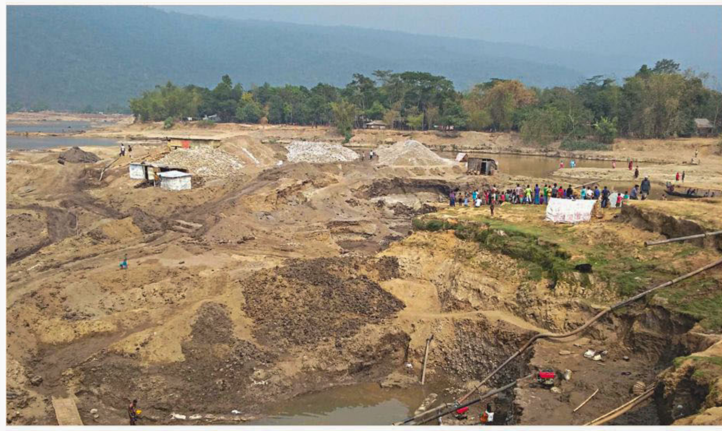
Defying a government ban, extraction of stones with dredgers from the Pyan river in Sylhet's Jaflong continues unabated. At least 14 workers have been killed in landslides during illegal stone extraction in Sylhet in the last two months. The photo was taken yesterday.
