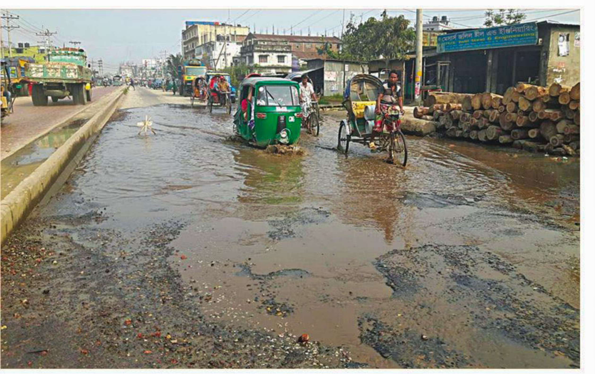
An overflow of sewage submerges part of Hemayetpur-Shingair road in the absence of proper drainage system, damaging the newly repaired road and posing serious hazards to pedestrians and vehicles. The photo was taken from Nazimnagar area on Tuesday.
