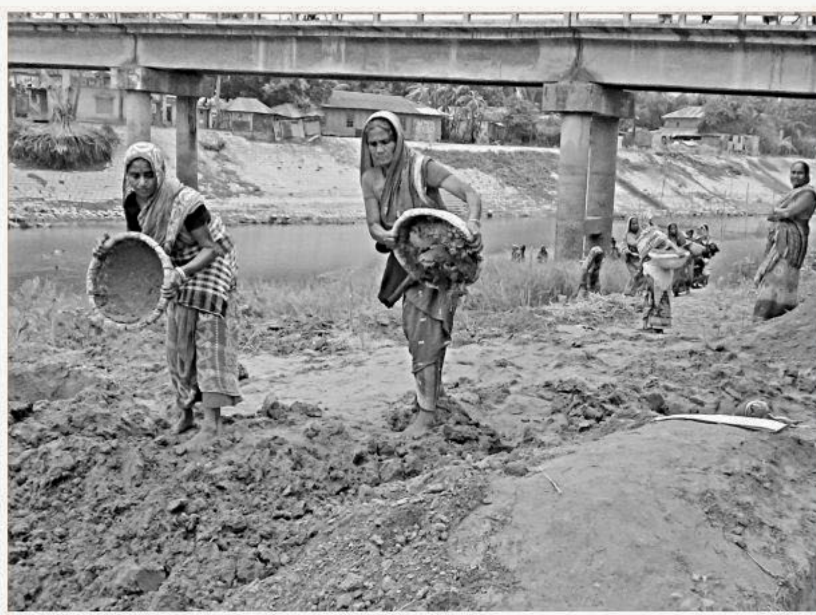
Workers, allegedly being paid by the government's "Employment Generation Programme for the Poorest", building the Jubo League office on the bank of the Barnoi river.
