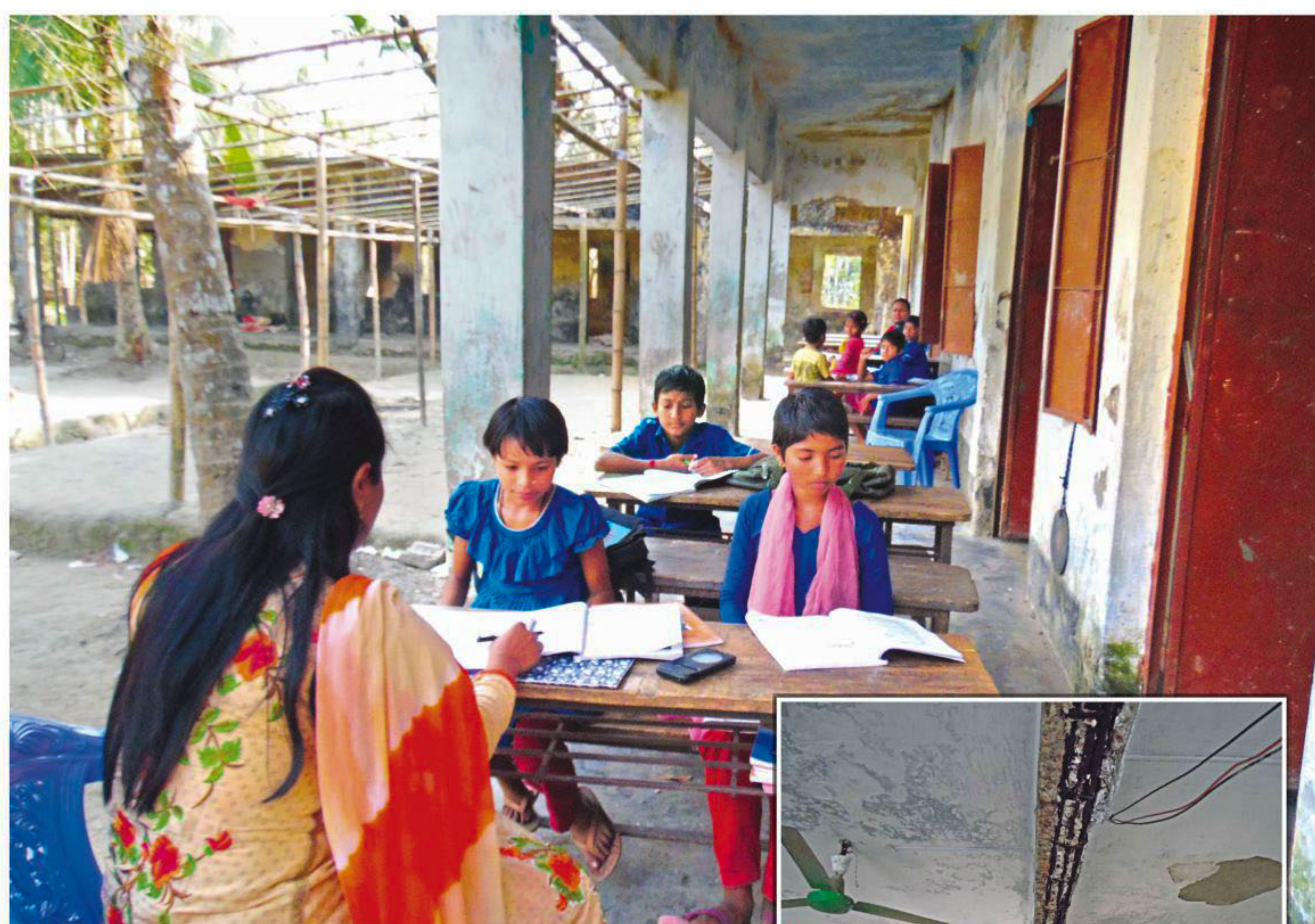
A teacher giving lessons to students on the verandah of dilapidated Jagodishpur Primary School building in Jhalakathi sadar recently. Many parents do not send their children to the school fearing it might collapse on them.
