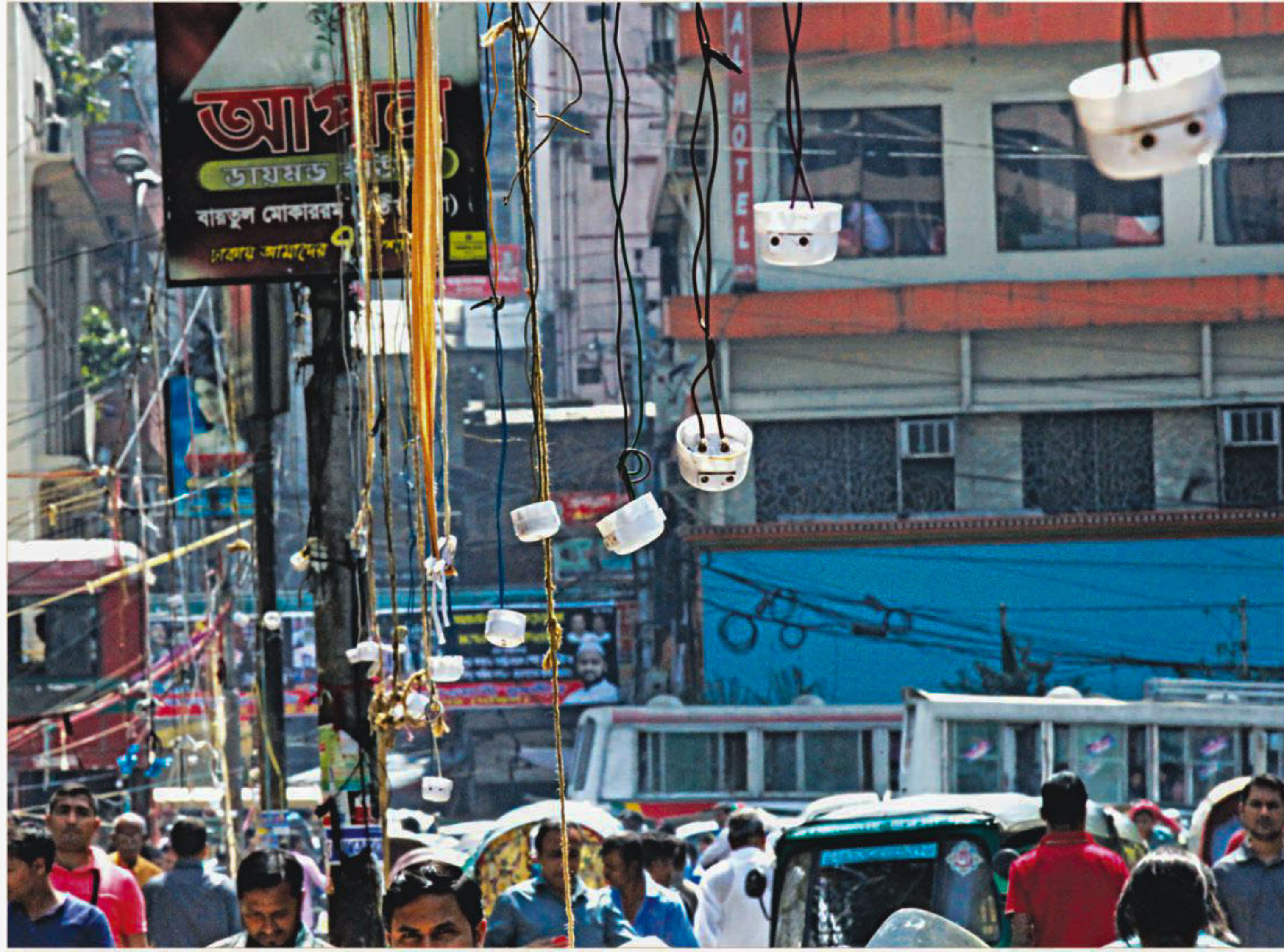
Power outlets hanging dangerously low over a pavement near the GPO in the capital yesterday. Hawkers use them while selling goods after hours and on Fridays.
