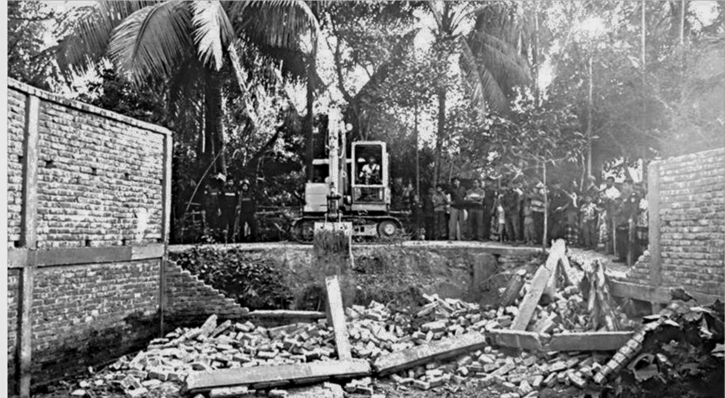
Paikgachha upazila administration demolishing a wall built by lawmaker of Khulna-6 constituency Sheikh Nurul Haque around the house of a local Awami League leader. The wall was erected over a land dispute in January 2016. Since then, the family had to use ladders to cross the boundary wall while holes were dug underneath so that elders and children can pass through. The issue came to light after the media reported on it recently.
