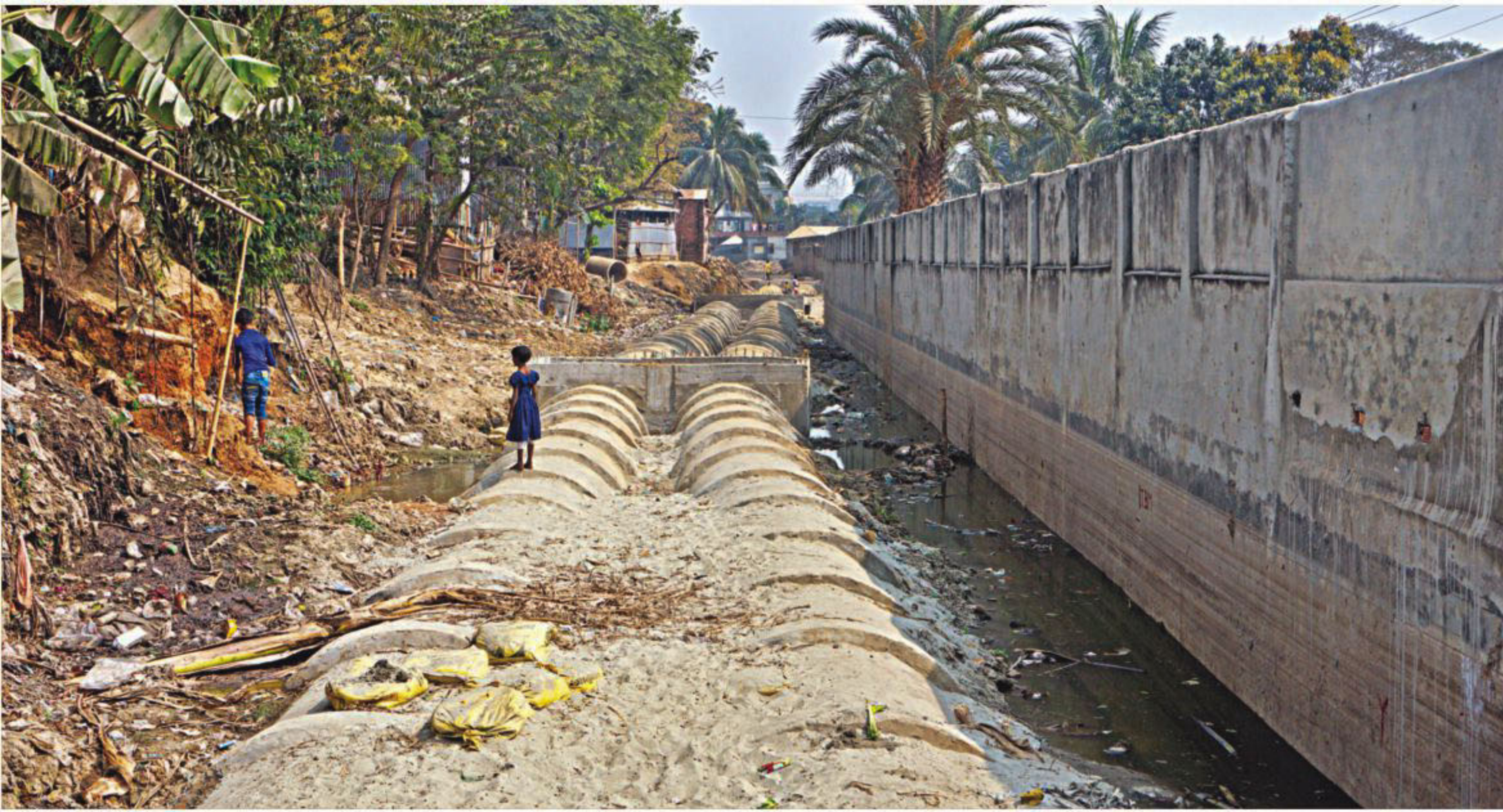
Sewer pipes being laid by the Savar municipal authority through a canal in Namabazar as per their initiative to mitigate the area's waterlogging crisis. The waterway, which used to flow into the Bongshi river, was already in dire straits due to unabated encroachment on its both sides with influential locals erecting boundary walls on one side and people building shanties on the other, narrowing it down considerably. Simultaneously, incessant dumping of waste continues to pollute the water body and exacerbates the drainage congestion. The photo was taken recently.
