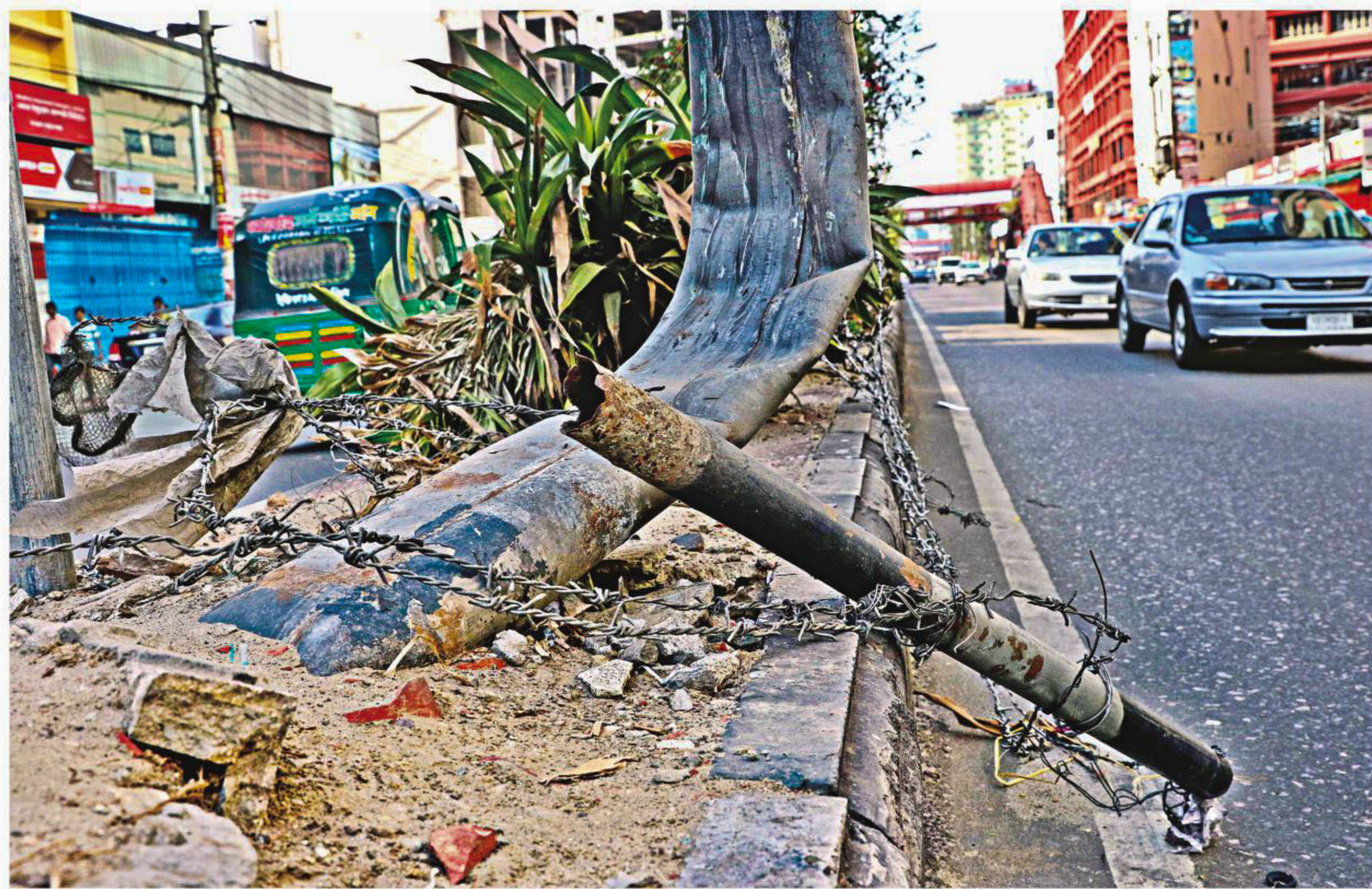
A bent electricity pole and a knocked over fence post on the median strip of Kazi Nazrul Islam Avenue. A bus recently ran into the median strip at night and hit the pole but it was not fixed. The photo was taken yesterday.
