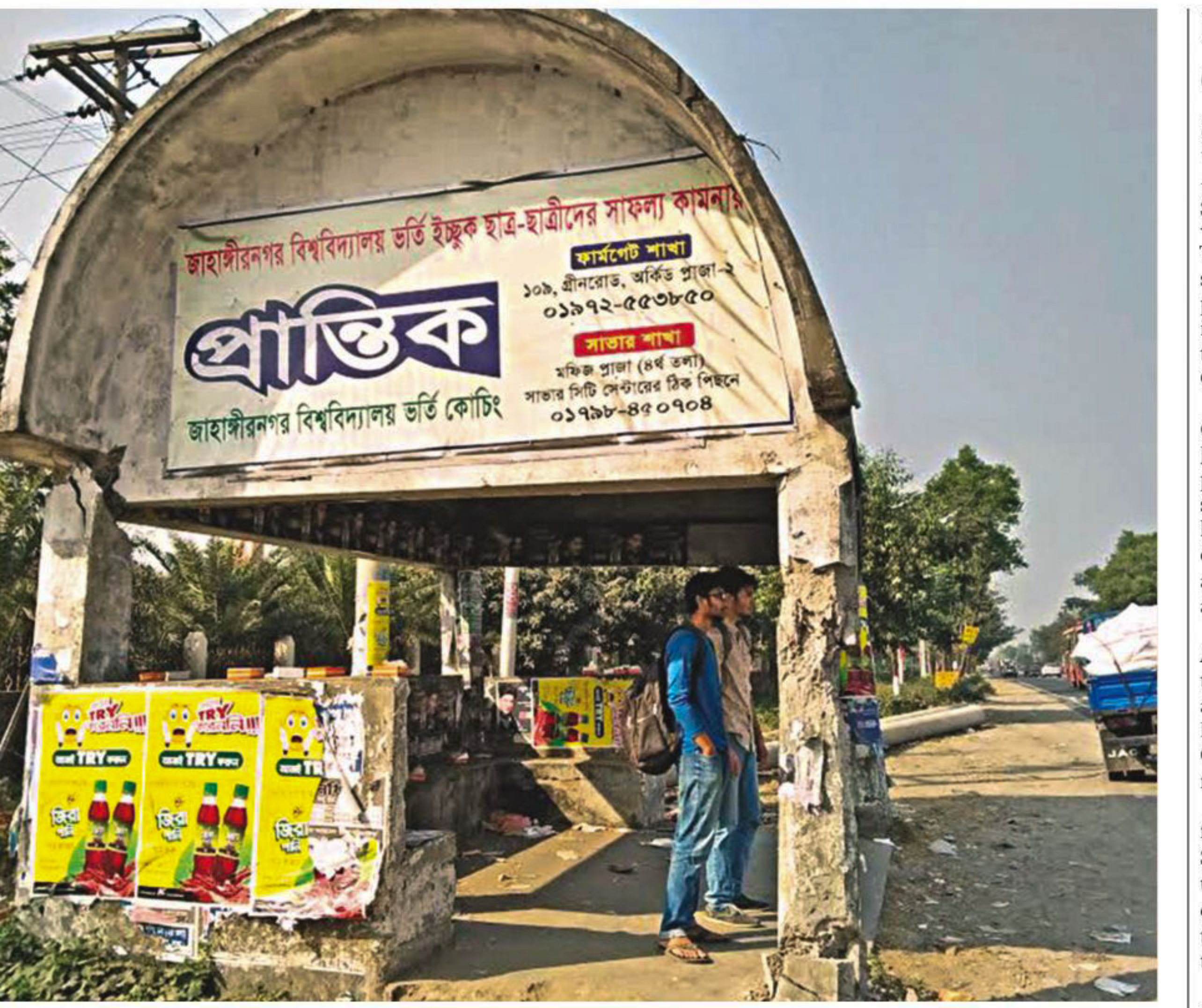
Students waiting for buses under the ramshackle passenger shed near Jahangirnagar University entrance. Though one month has already passed since a bus hit the shed while trying to overtake another, the authorities concerned are yet to take any initiative to repair it. The photo was taken recently.
