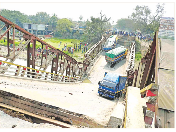
This bridge over the Chitra river in Magura's Simakhalo on Dhaka-Khulna highway collapsed yesterday when two lorries, two of them laden with stones, were crossing it. Two people on the bridge were injured. Traffic was diverted via Jhenidah following the incident.
