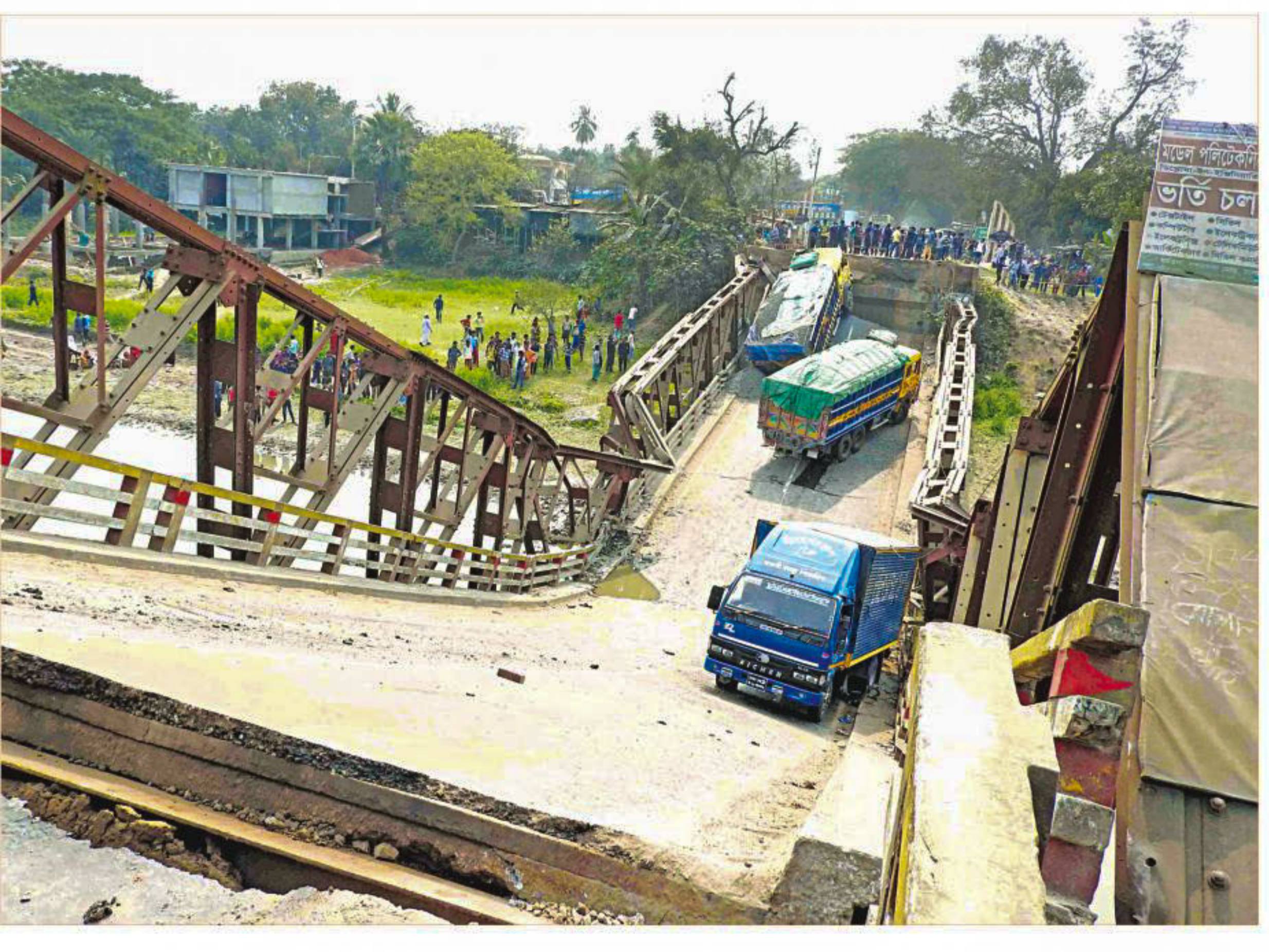
This bridge over the Chitra river in Magura's Simakhali on Dhaka-Khulna highway collapsed yesterday when three lorries, two of them laden with stones, were crossing it. Two people on the bridge were injured. Traffic was diverted via Jhenidah following the incident.
