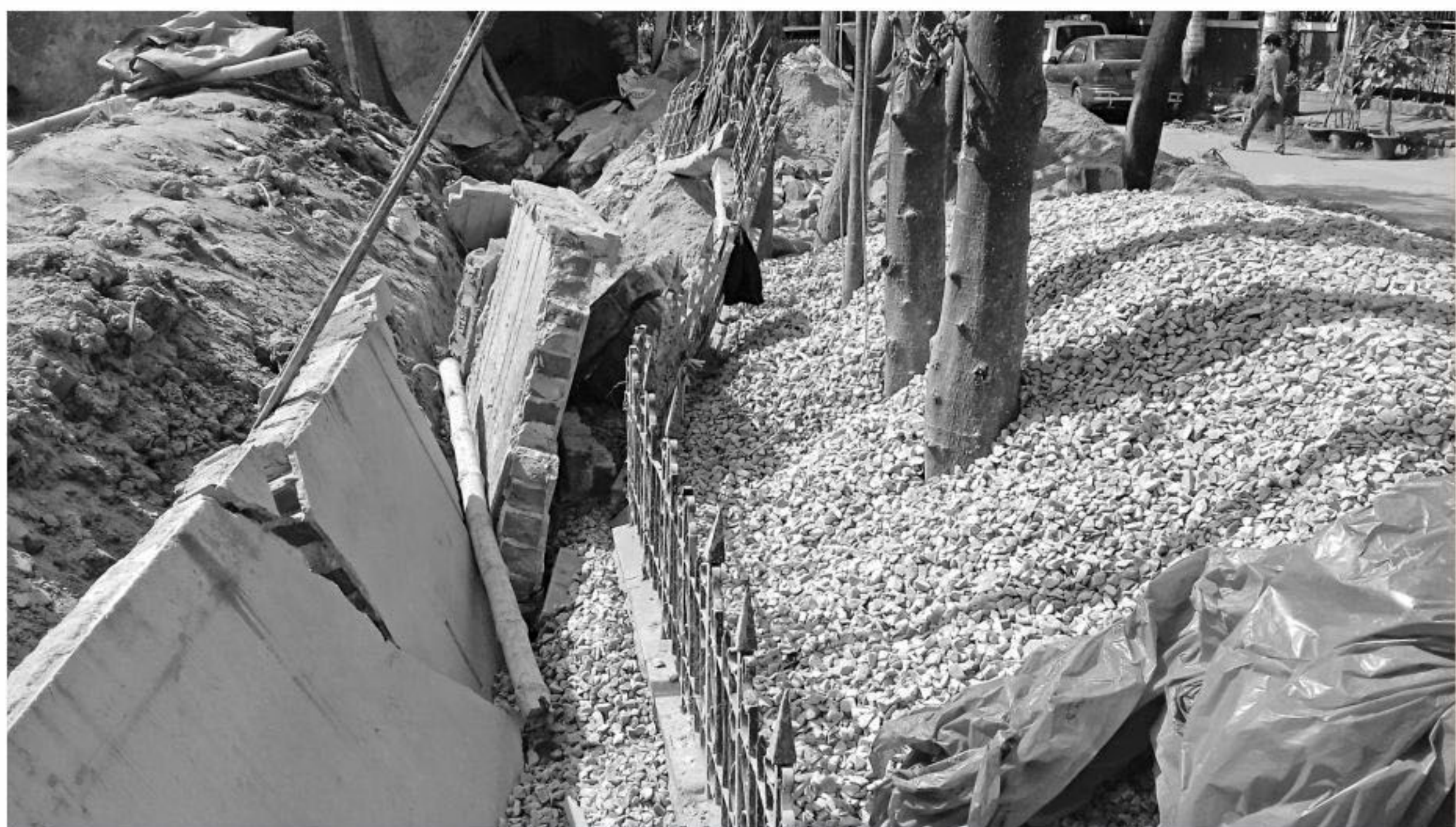
The wall in Baridhara in the capital that fell on four construction workers yesterday, killing a female labourer.
