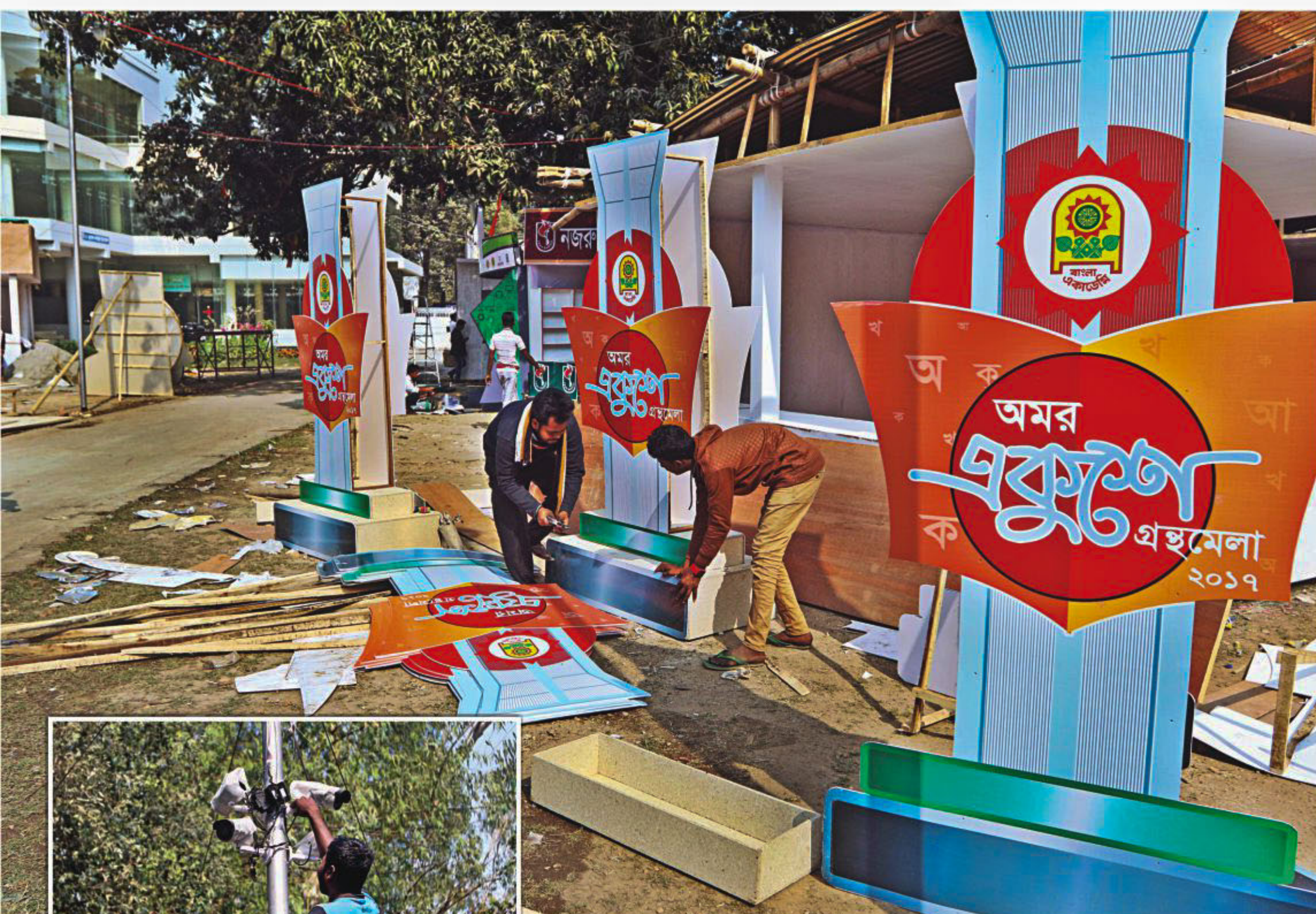
Book stalls are being built and CCTV cameras, inset, are being installed in and around the Bangla Academy yesterday where the month-long Amar Ekushey Book Mela is set to begin today.
