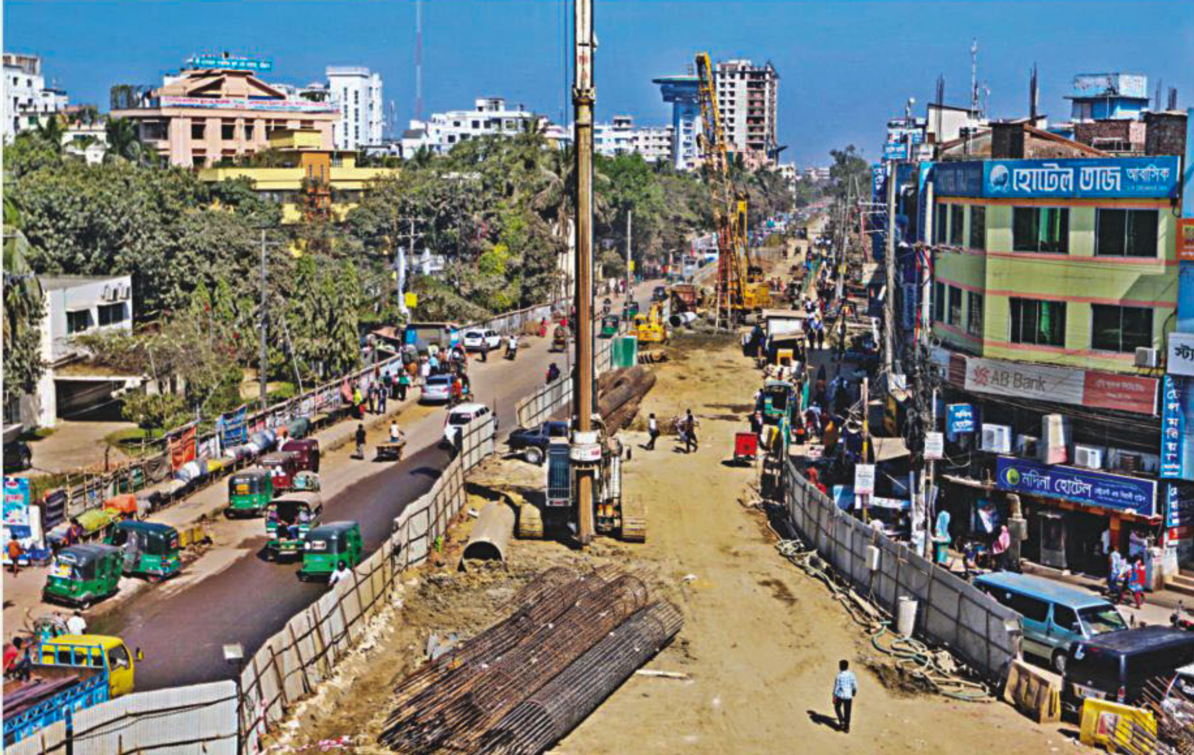
Works of Bahaddarhat-Muradpur flyover, initiated by Chittagong Development Authority, continuing on a section stretching towards Kalurghat after a portion of it collapsed on November 12, 2012. The photo was taken yesterday.
