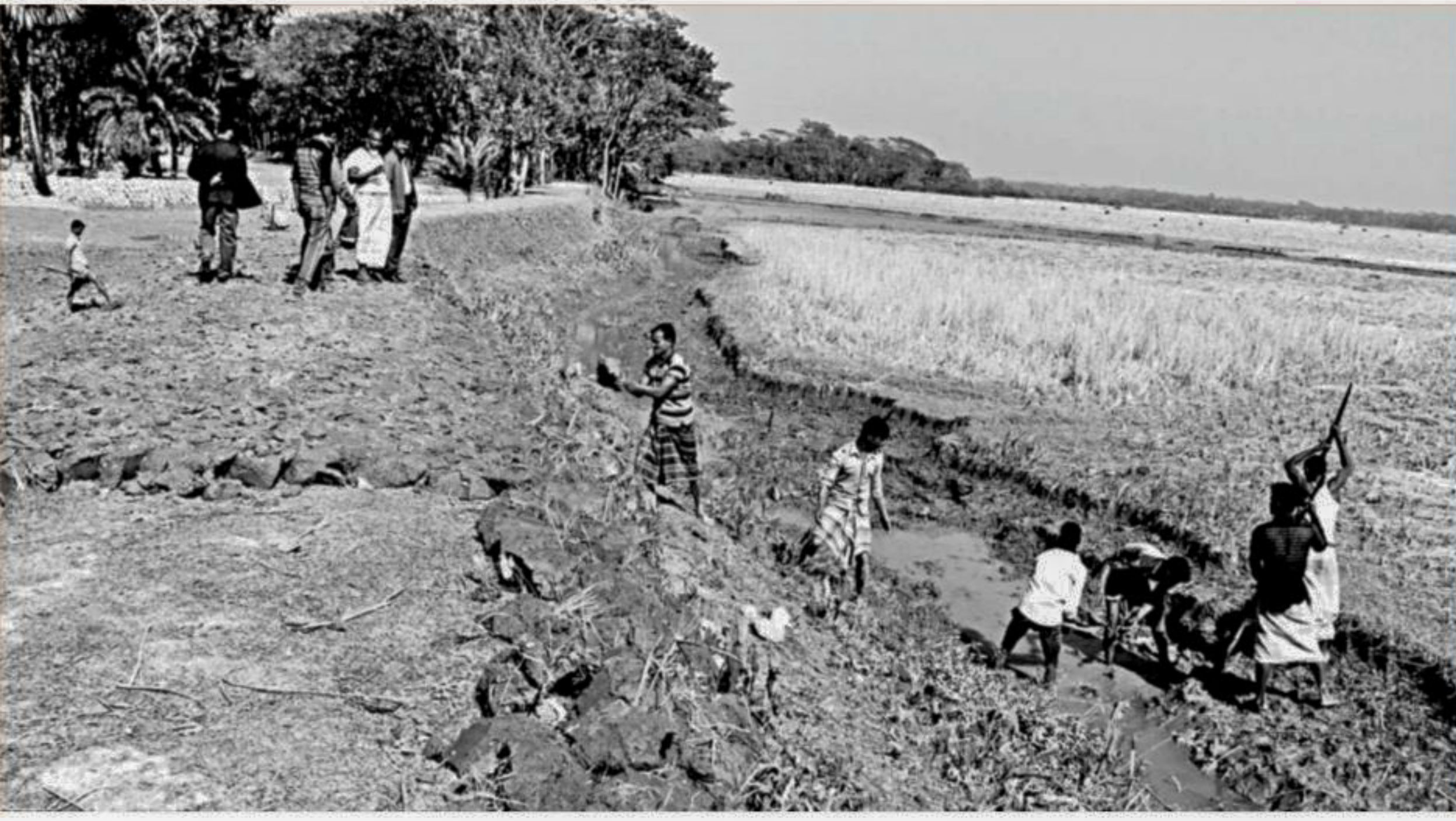
Villagers join hands to repair a one kilometre portion of damaged embankment to stop river erosion at Palat in Rajapur upazila of Jhalakathi.
