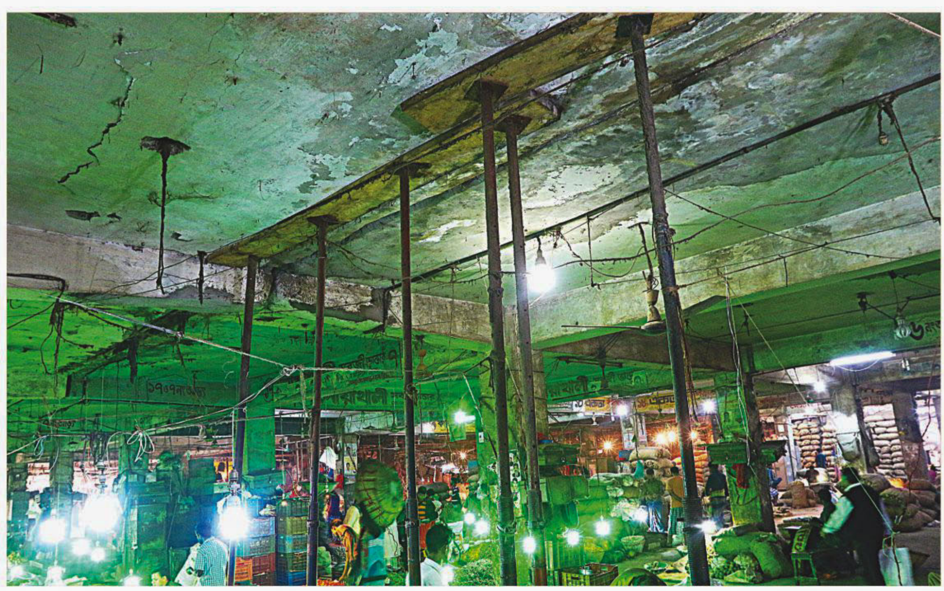
The ceiling of a building of the Karwan Bazar kitchen market is propped up by iron pipes to prevent any accident for the time being. But nobody knows how long the pipes are going to hold as the authorities of the market keep on adding more pipes with the condition of the heavily worn-out ceiling getting worse every day. A major wholesale hub of the capital, the market is frequented by buyers and traders almost round the clock and any major accident is likely to result in huge casualties. The photo was taken Sunday. PHOTO: PALASH KHAN
