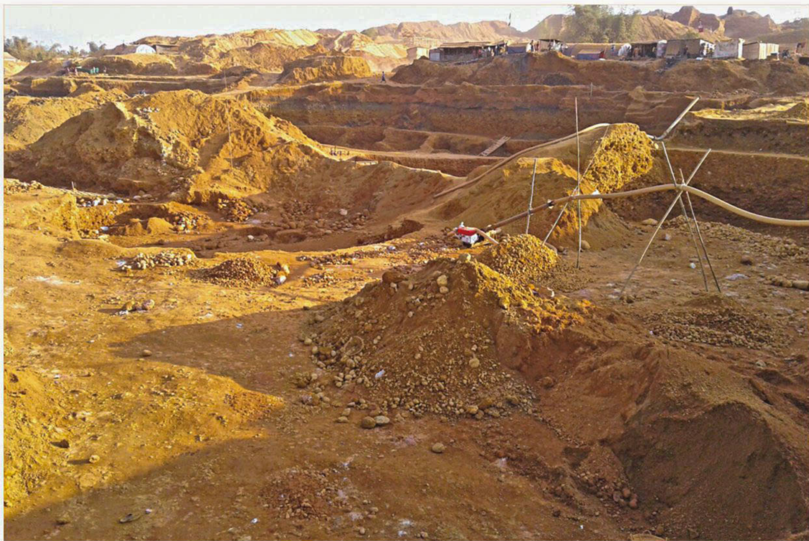
The part of Shah Arefin Tila where two workers were killed in a landslide while extracting stone. The photo was taken yesterday.
