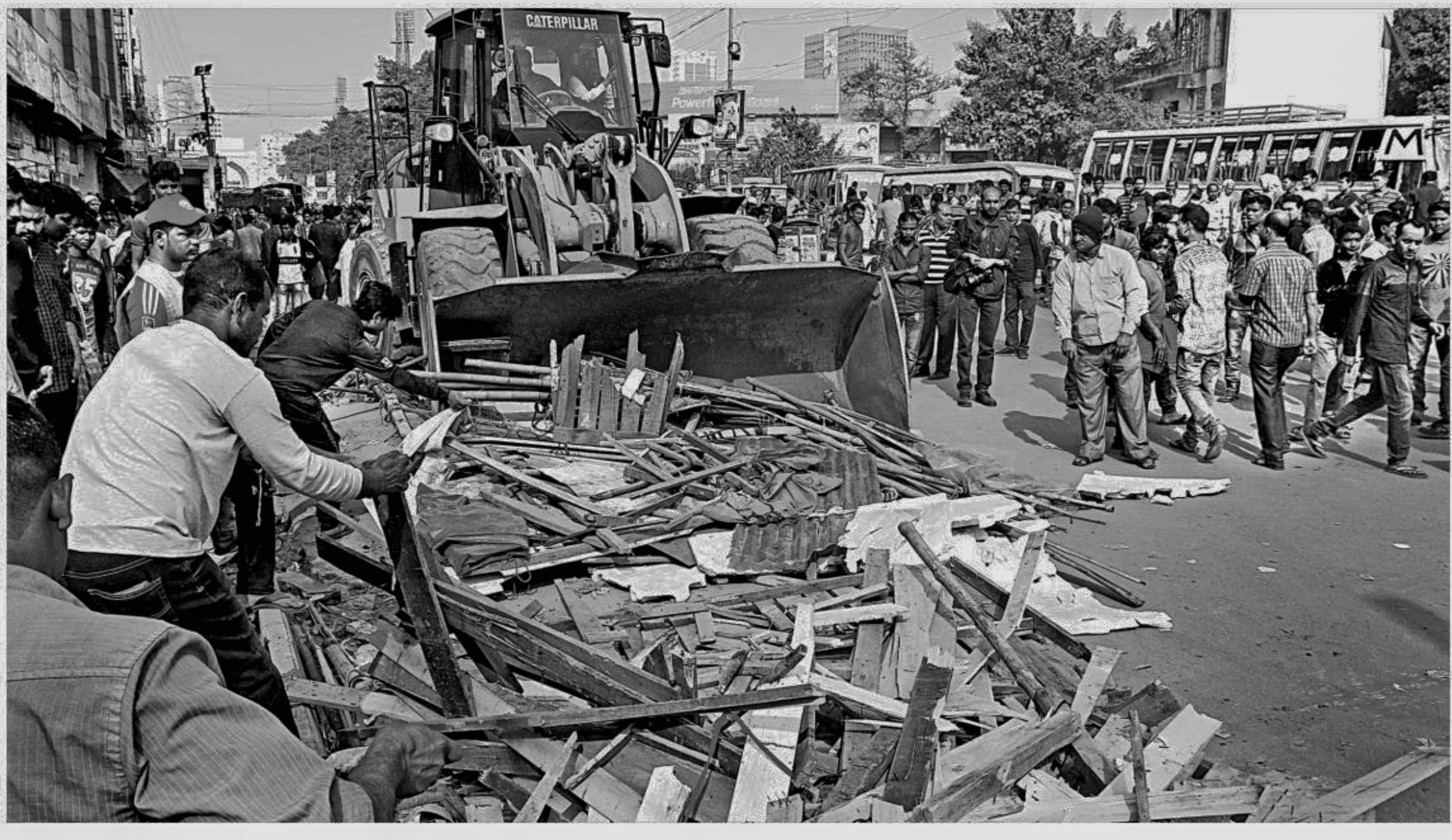
Dhaka South City Corporation authorities demolish illegal structures in the capital's Gulistan yesterday to free the footpath from hawkers. The photo was taken around 2:00pm.
