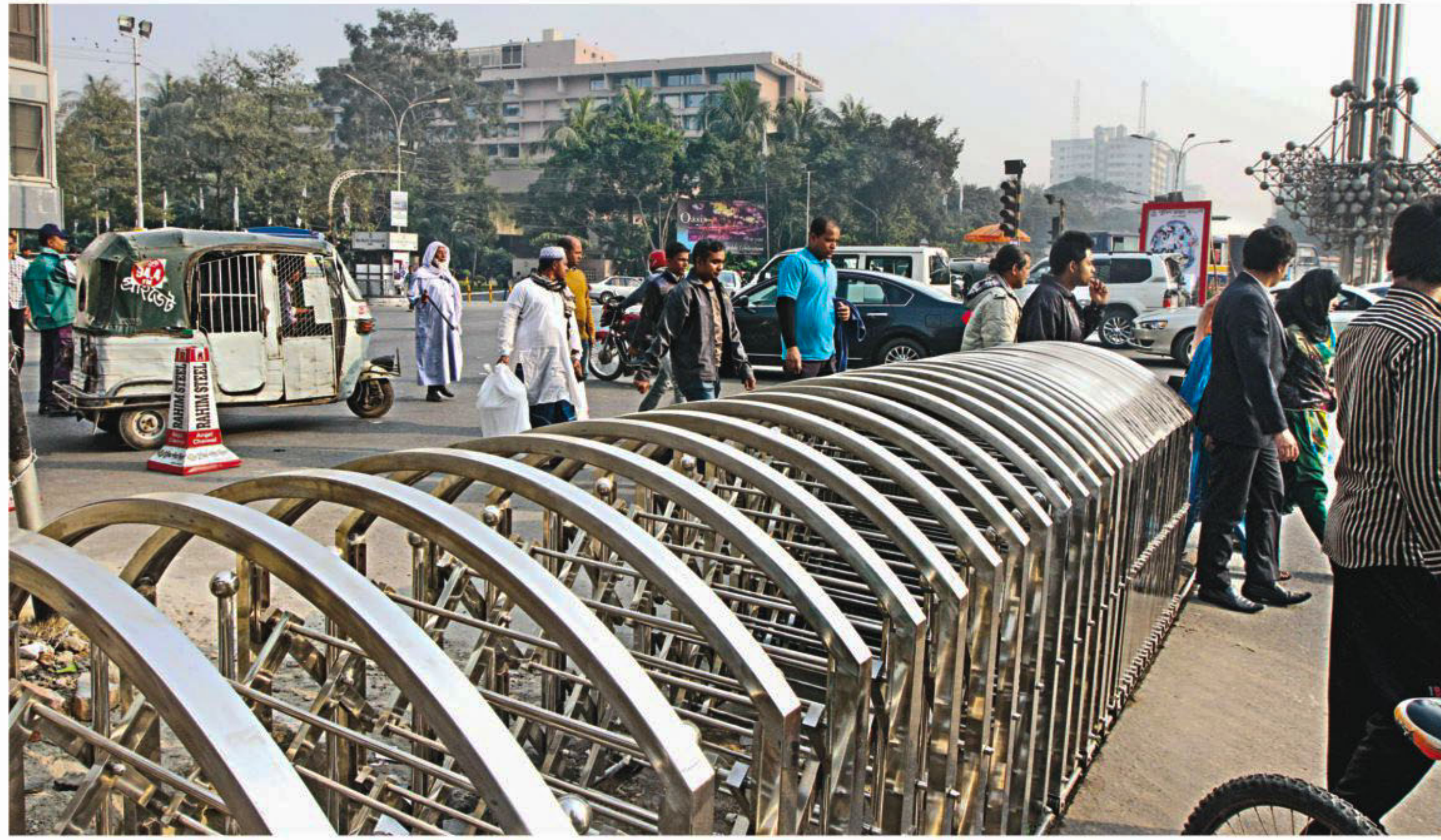
A folding barrier is being installed at the capital's Sonargaon intersection by Dhaka North City Corporation to control traffic and stop jaywalking. A traffic sergeant yesterday said they would initially use the barrier during movement of VIPs through the area. PHOTO: SK ENAMUL HAQ
