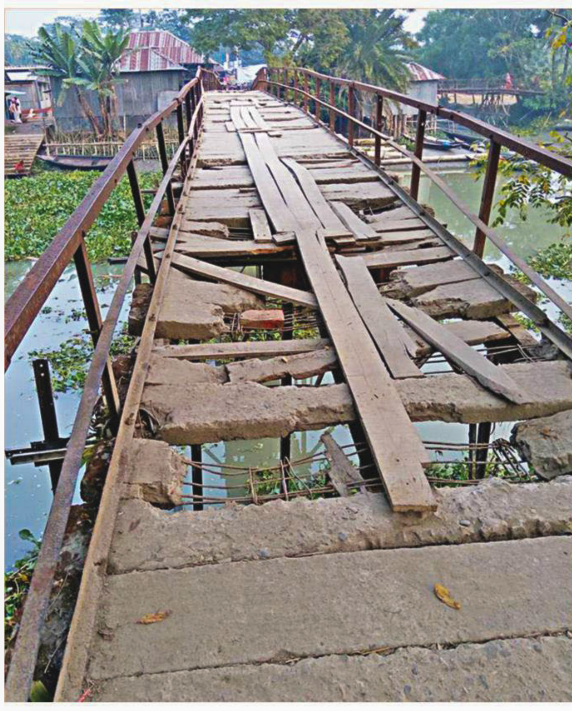
The rundown iron bridge on the Sandhya river's branch in Udoykathi union under Banaripara upazila of Barisal. PHOTO: STAR
