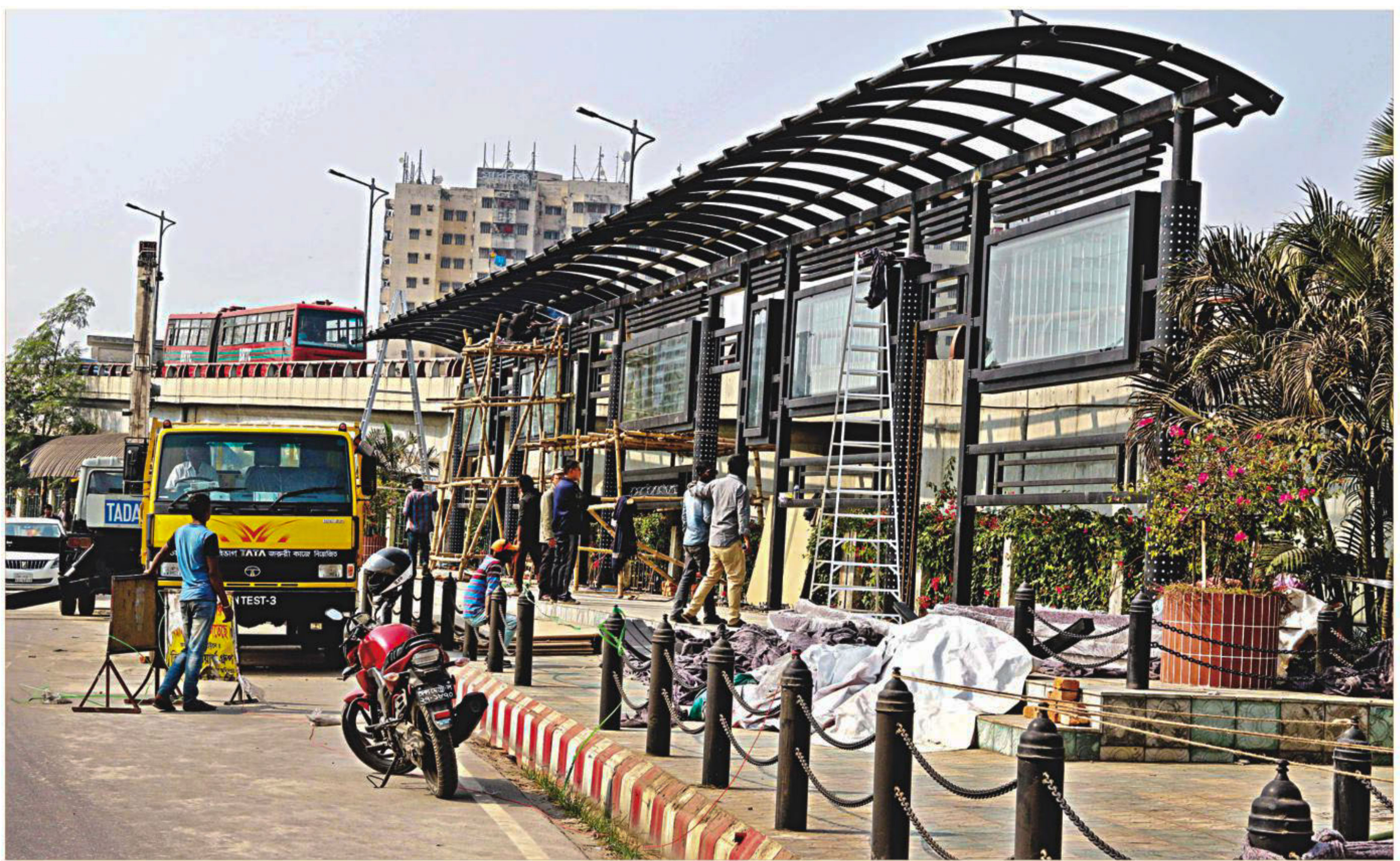
Work goes on in full swing for the country's first ever digitalised passenger shade next to the capital's Airport Road near the Cantonment area. The 135ft stop area will also feature LED displays making people aware of road safety among others. The photo was taken yesterday.
