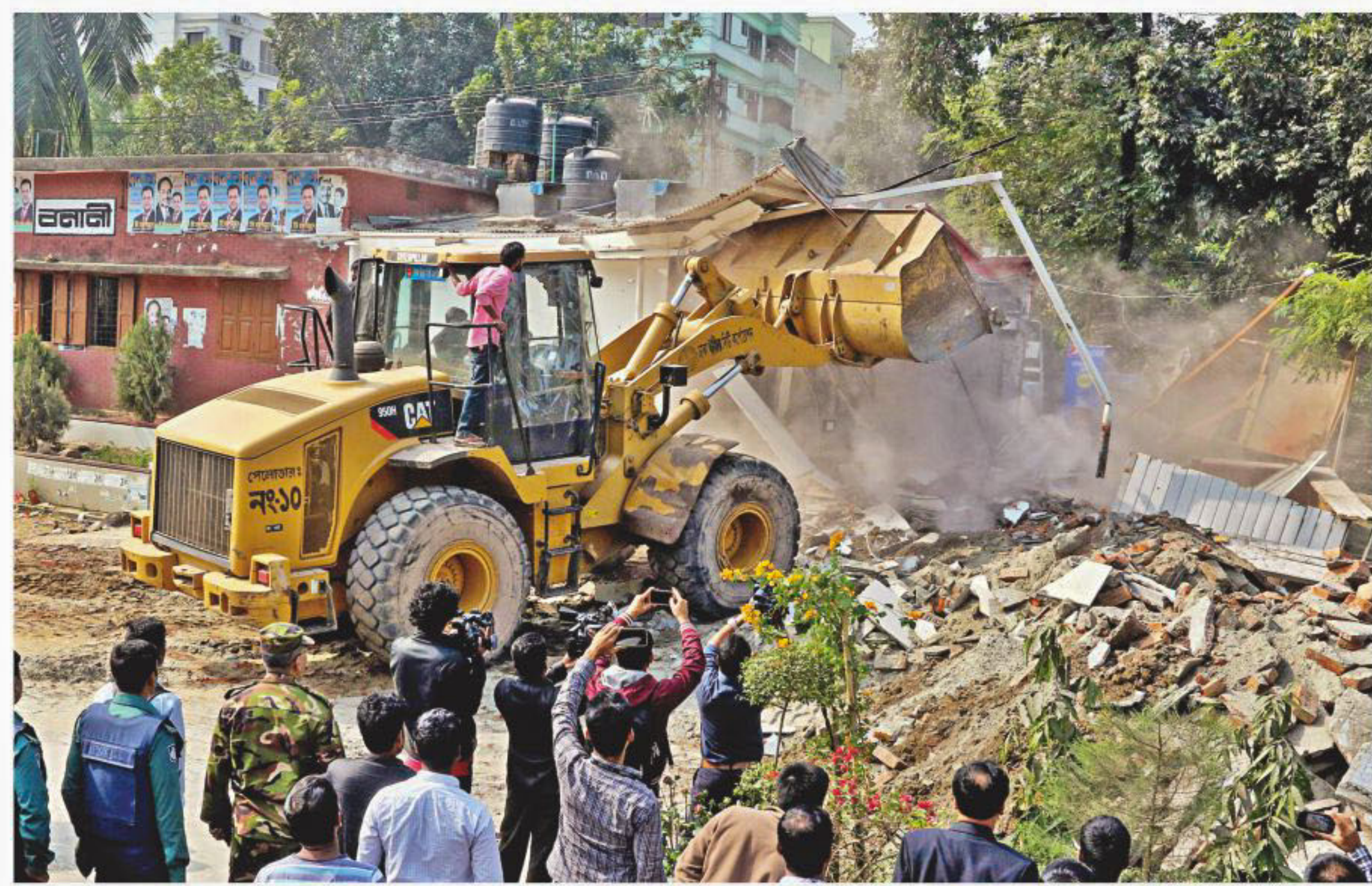
A Dhaka North City Corporation bulldozer knocks down an illegal structure on railway's land near the capital's Banani Railway Station yesterday. During the drive, the DNCC demolished over 2,000 such establishments, including Tehari on Wheels restaurant and parts of Banani Fast Food, in Mohakhali and Banani areas. PHOTO: ANISUR RAHMAN
