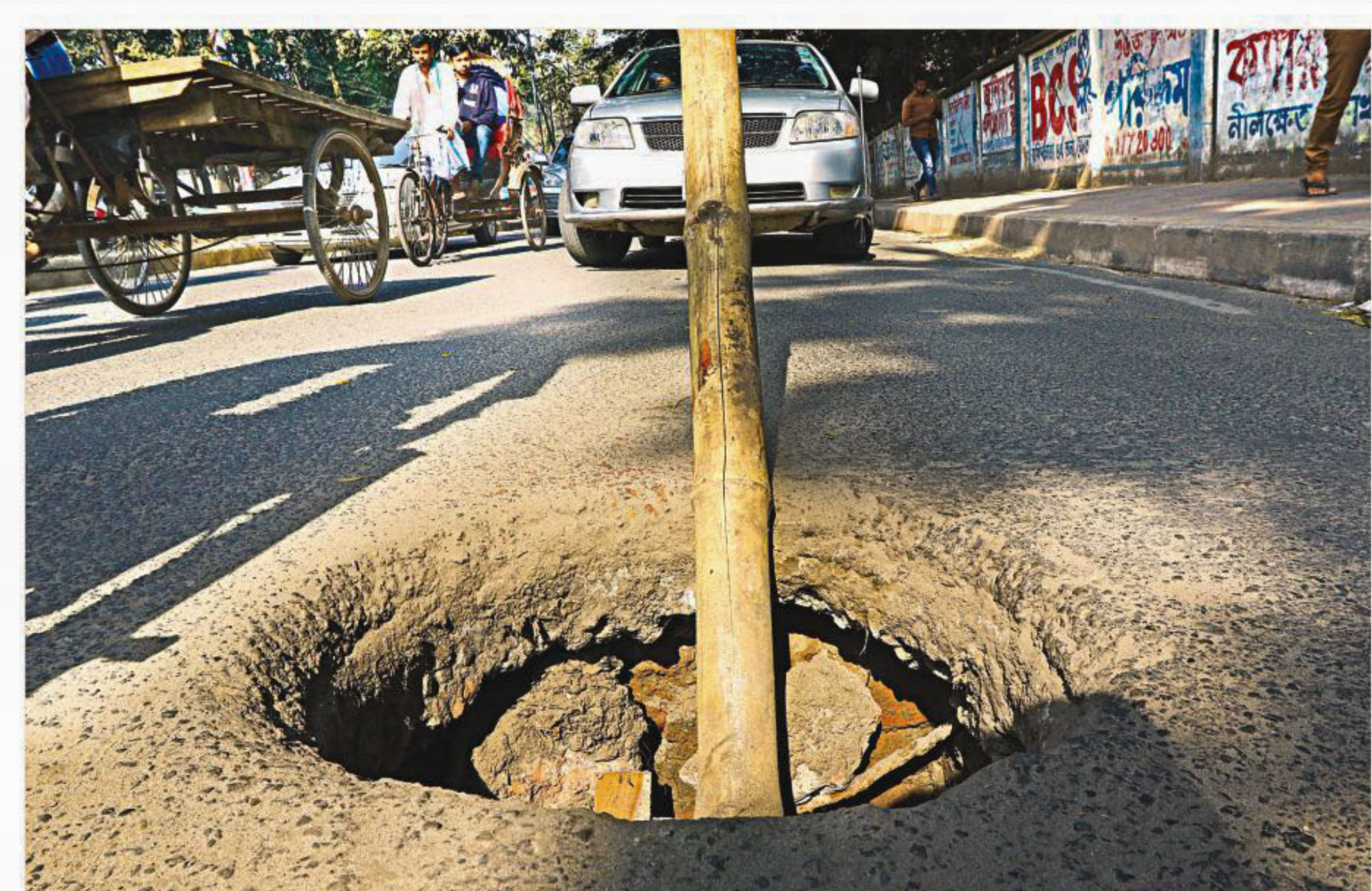
A bamboo pole serves as a warning for a sewer opening on the road opposite Newmarket Police Station in the capital, posing the risk of an accident for oncoming traffic. The photo was taken on Saturday.
