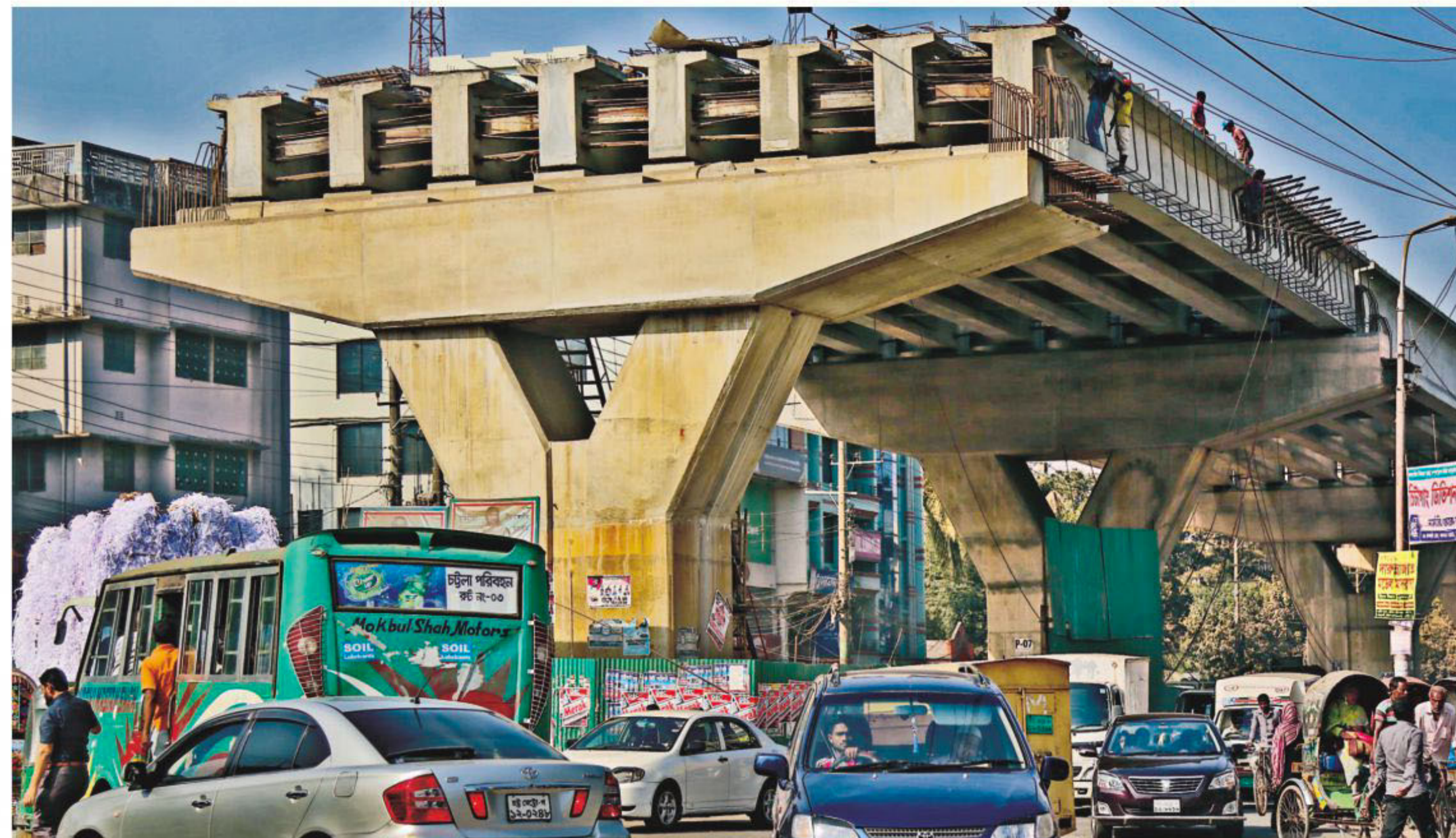
Absence of adequate safety measures has resulted in an iron rod falling off this under-construction flyover stretching from Muradpur to the Ispahani intersection in Chittagong city on Sunday evening, damaging a car passing underneath. On June 29, 2012, a rickshaw-puller made a lucky escape with just bruises after a concrete girder of another flyover at Bahaddarhat, then under-construction, collapsed.
