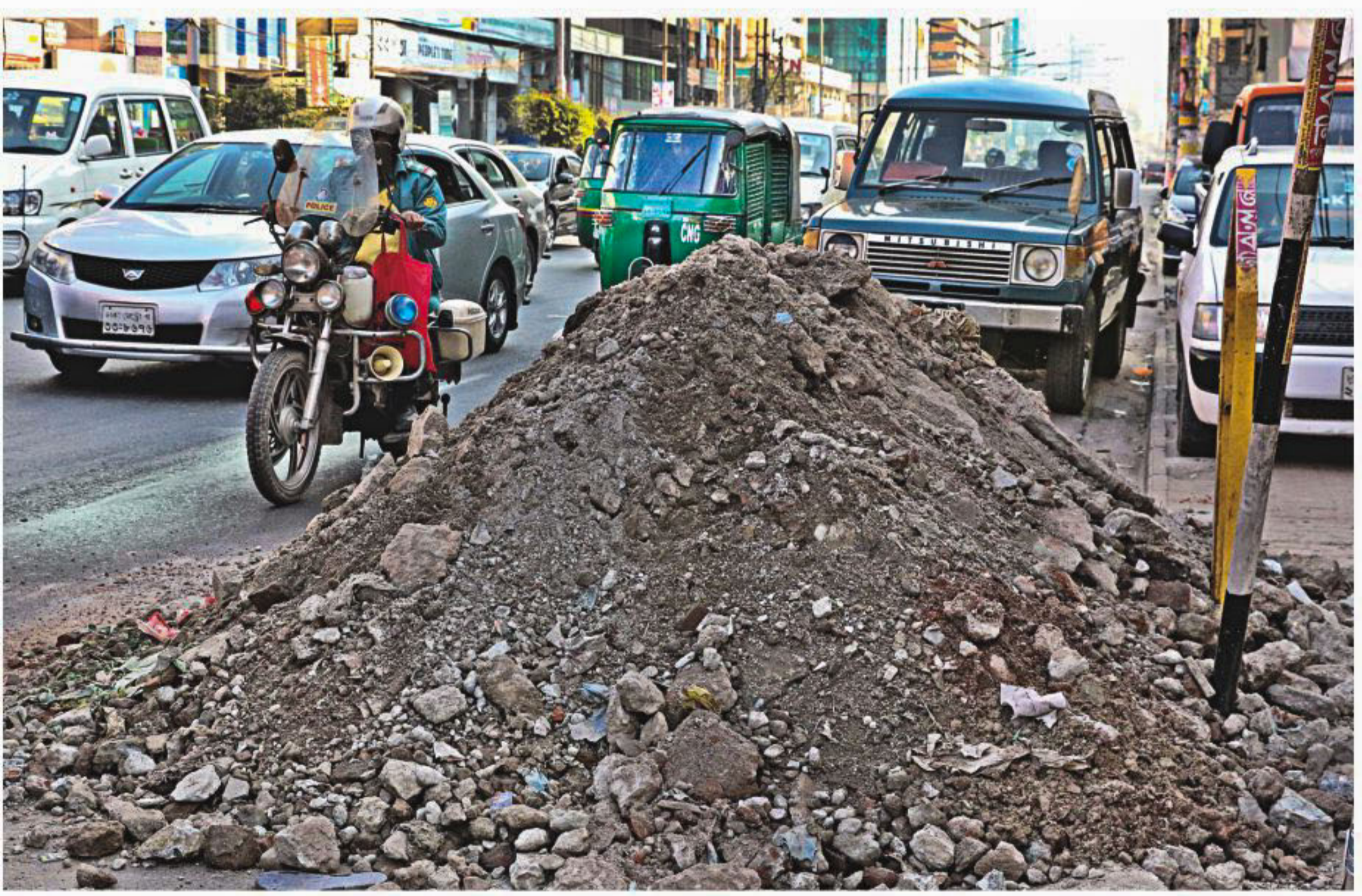
Traffic on Kazi Nazrul Islam Avenue gets obstructed for earth piled up from road development works being carried out by Dhaka North City Corporation in East Tejguri Bazar in the capital. The photo was taken around 2:30pm yesterday.
