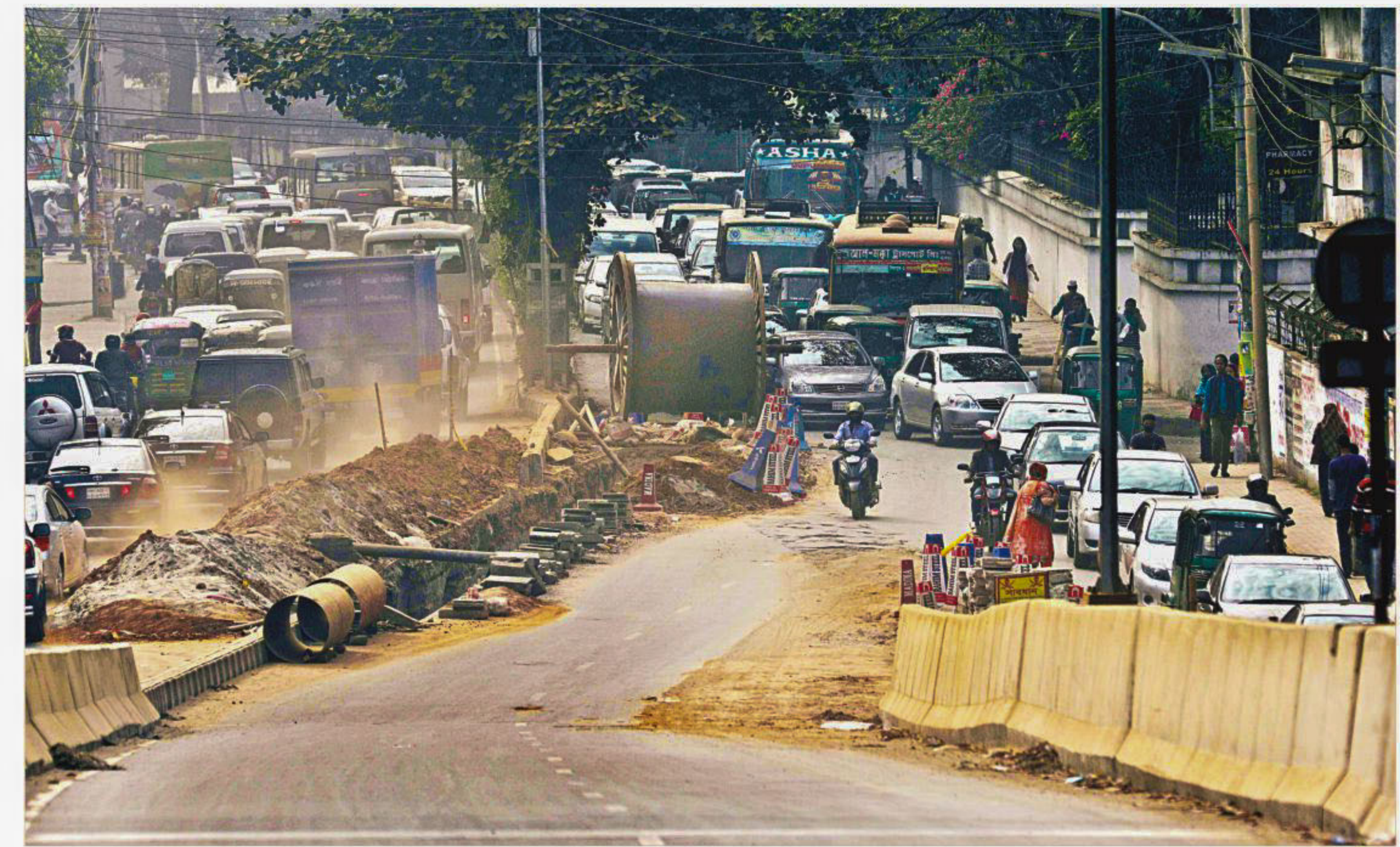
A cable reel and earth, dug out for underground electricity line, kept on the slope of Moghbazar-Mouchak flyover on Shaheed Captain Mansur Ali Sarani in Dhaka, contributing to traffic jam yesterday.
