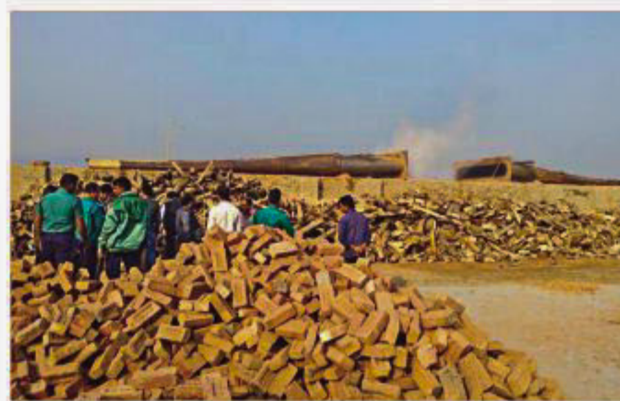
Two drum chimneys lie on the ground at Doarika in Babuganj upazila of Barisal after a mobile court of the Department of Environment knocked them down during an ongoing special drive against illegal brick kilns recently.
