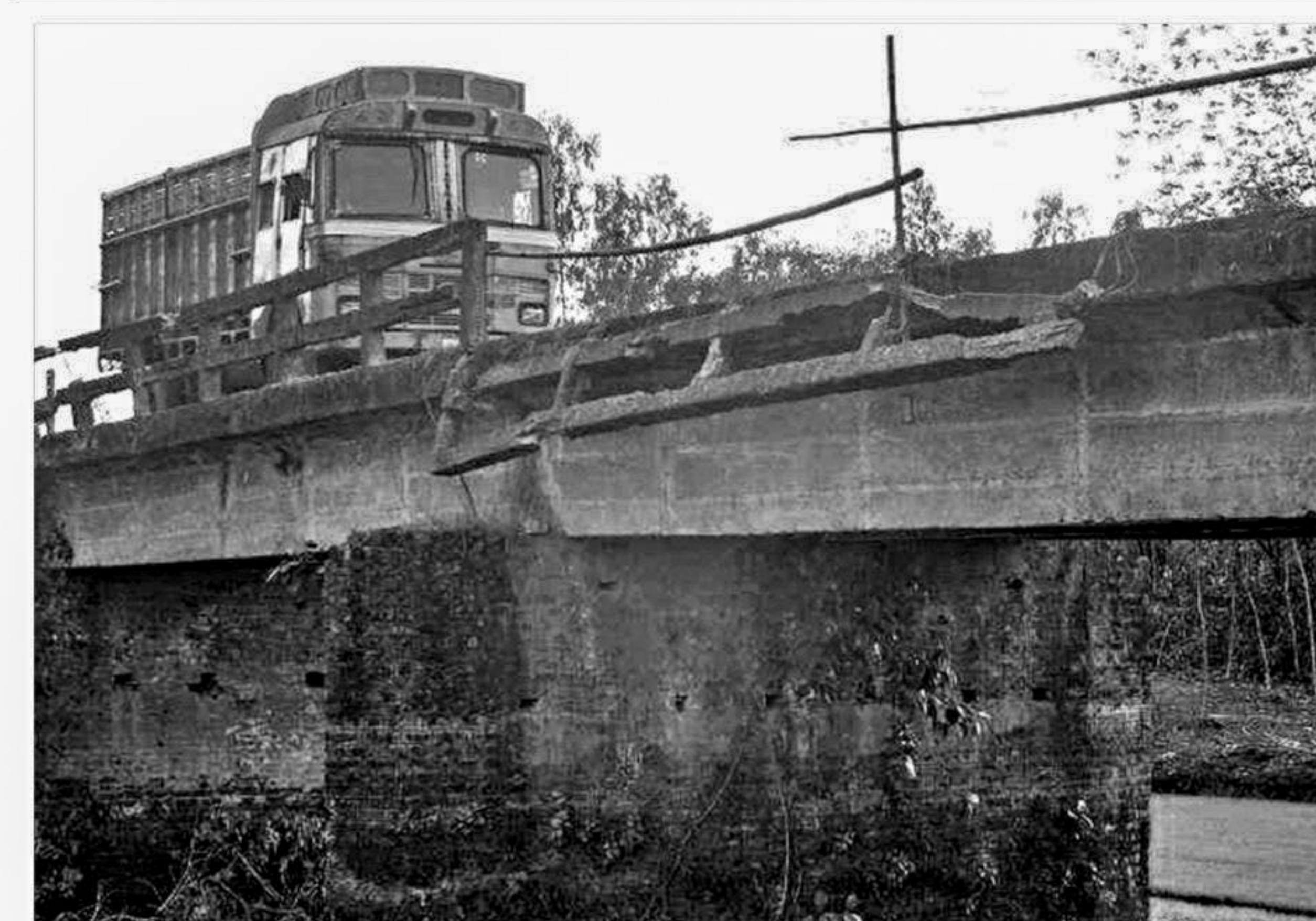
Vehicles cross this bridge at Kochua point on Nilphamari-Panchagarh road at great risk as its pillars have developed big cracks and the railings are breaking up.
