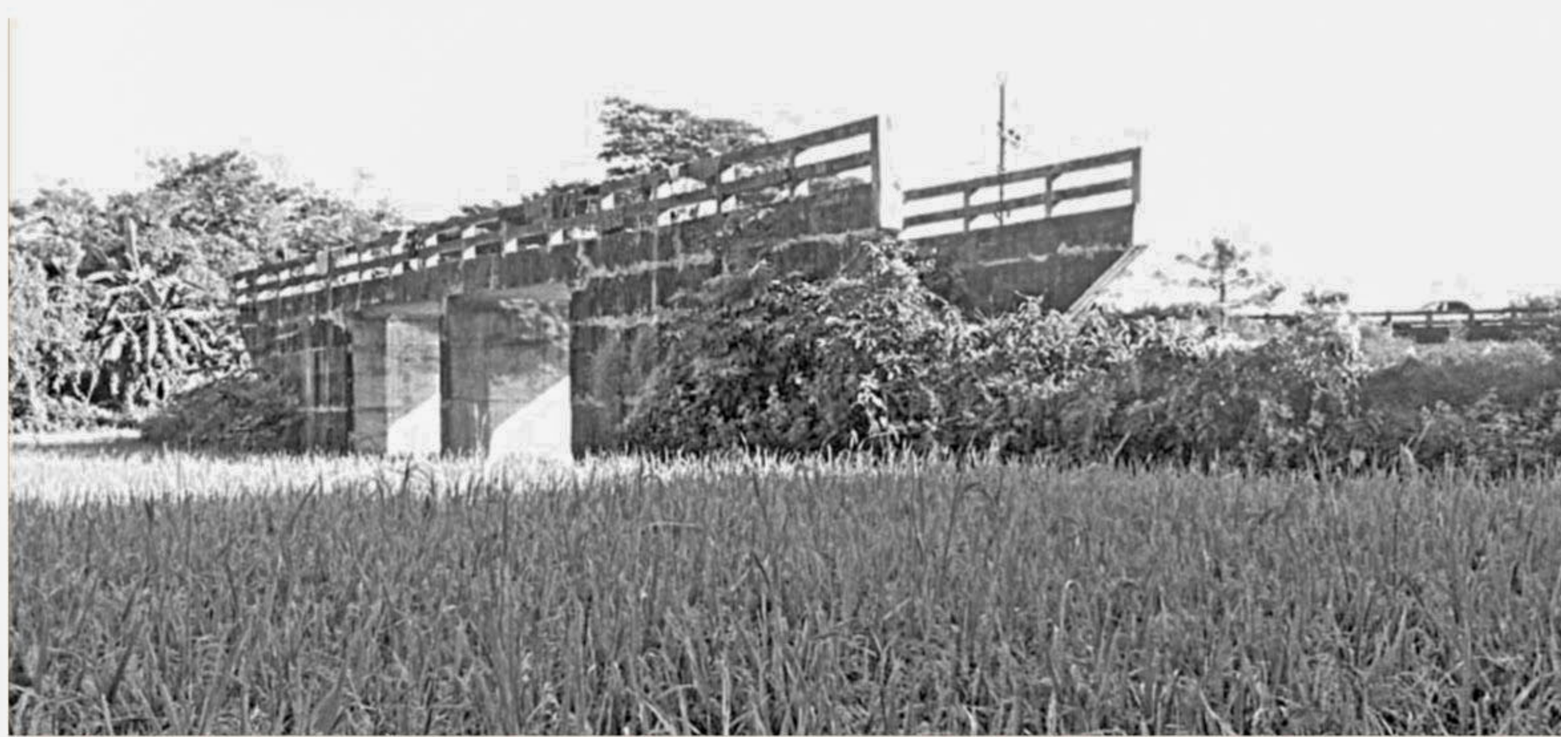
This concrete bridge at Khoinkut village in Narsingdi's Shibpur upazila remains useless for locals since completion of its construction more than a decade ago as it cannot be used due to lack of connecting roads. PHOTO: BENAJIR AHMED
