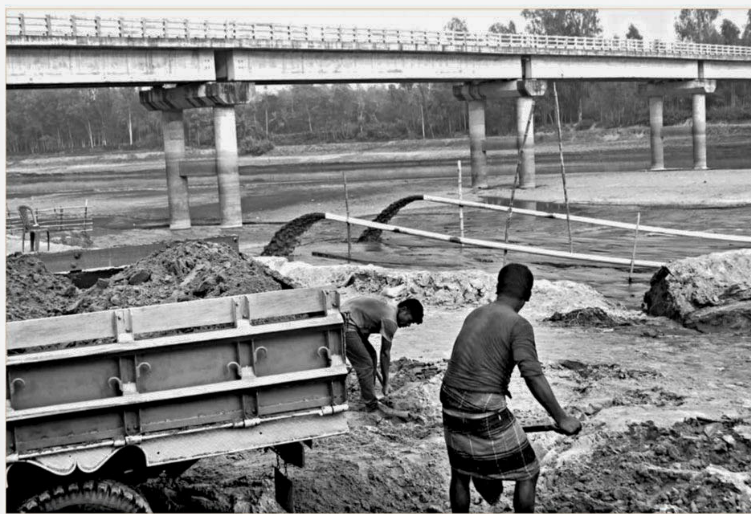
An influential local has been illegally lifting sand with dredgers in Bererbari area of Nimgaci union under Dhunat upazila of Bogra, threatening the nearby bridge over the Bangalee river and farmlands and homesteads in the area. PHOTO: STAR
