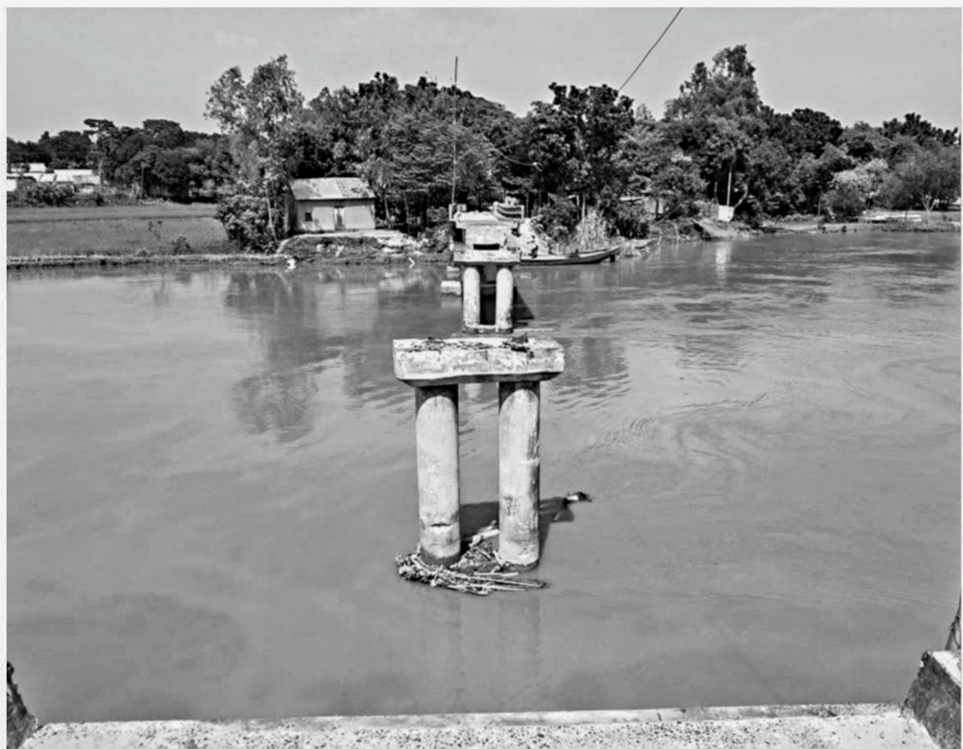
CLOCKWISE FROM LEFT: The collapsed bridges over the Jhinai river at Kajirpara in Basail upazila under Tangail and Dola canal on Mirganj-Khutamara road in Jaldhaka upazila of Nilphamari, and the awfully risky bridges on Kedarpur canal in Babuganj upazila under Barisal and a canal near GK High School in Rajapur upazila under Jhalakathi.
