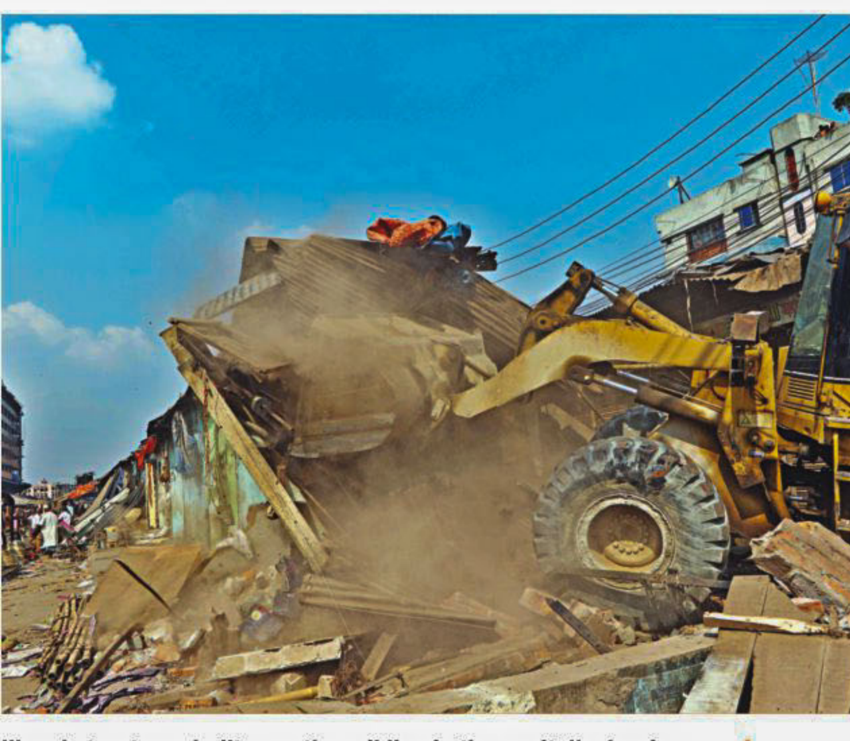
Illegal structures built near the rail line in the capital's Jurain being bulldozed yesterday. PHOTO: PRABIR DAS
