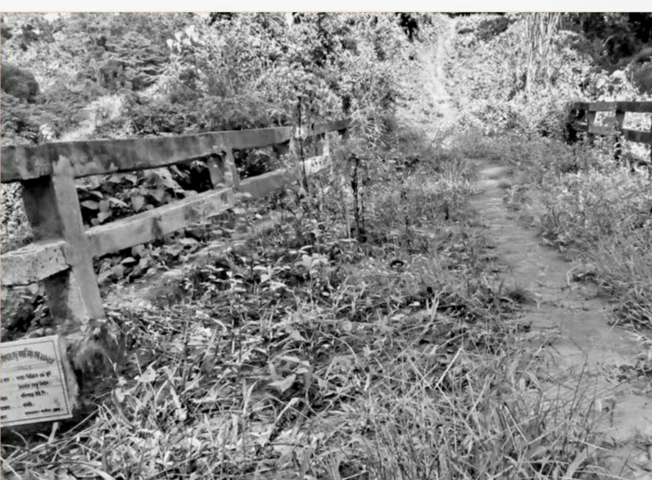
This patch of wild weeds and bushes is actually a 39-foot long bridge over a hilly spring (locally called chhara) in Bolipara under Thanchi upazila of Bandarban. Built by the disaster management ministry in 2014 at a cost of Tk 40 lakh, it is rarely used by the locals.
