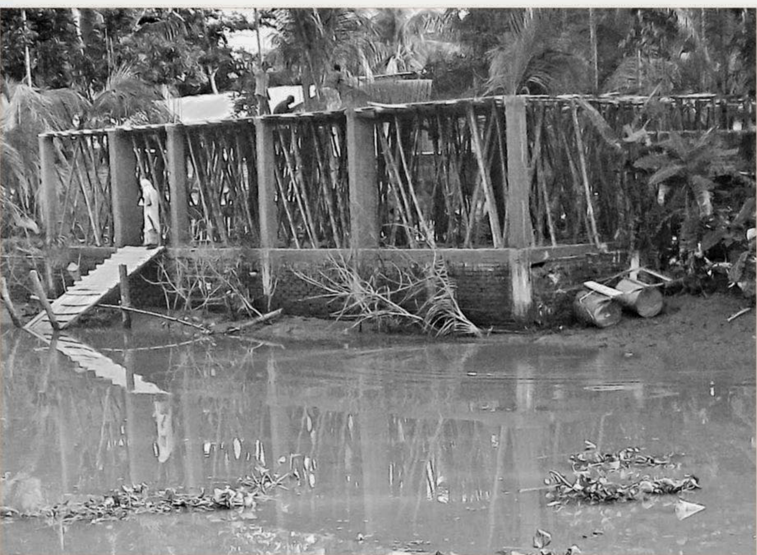
A building is being constructed encroaching on a canal at Dashpara in Baufal upazila headquarters of Patuakhali.
