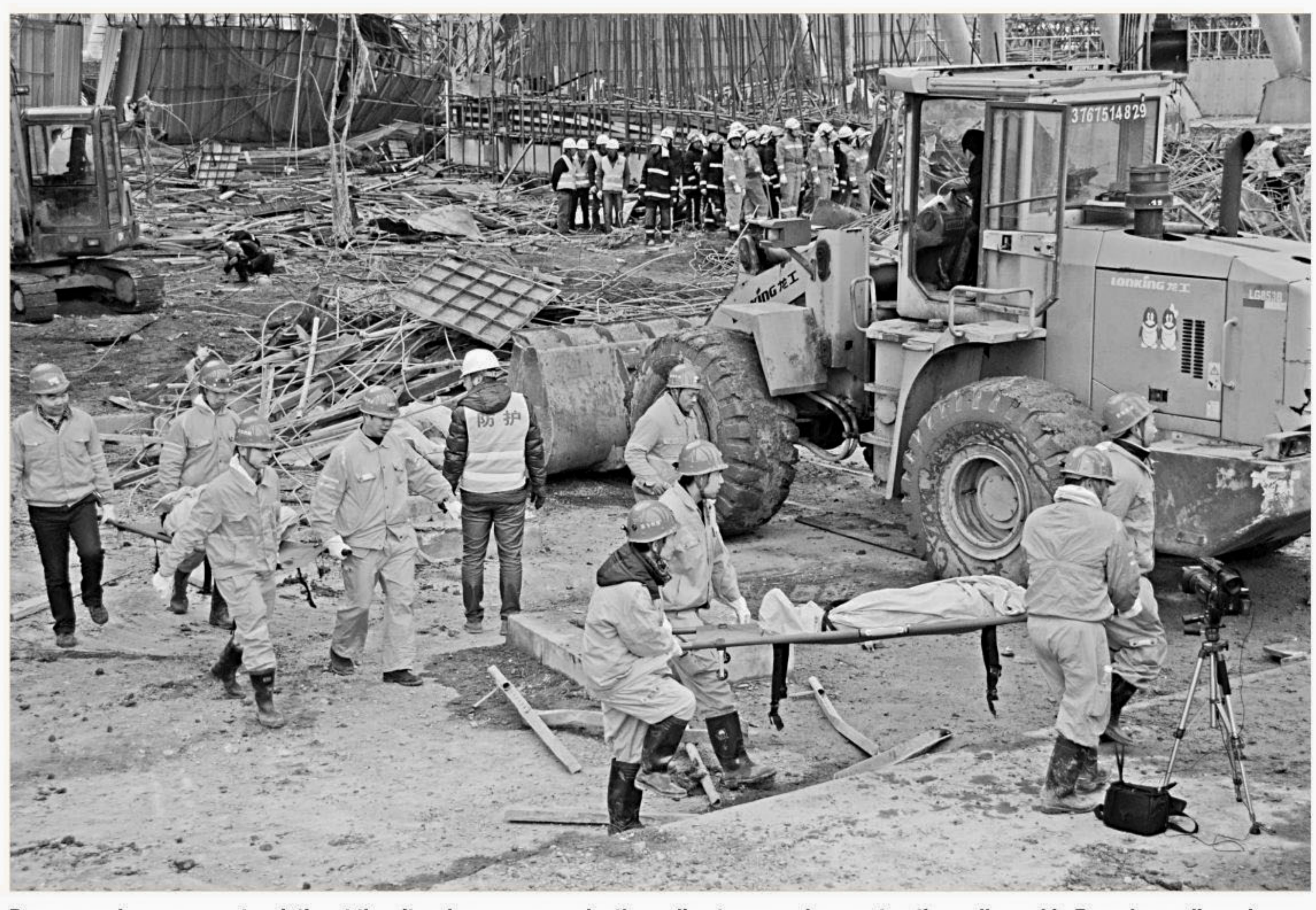
Rescue workers carry out a victim at the site where a power plant's cooling tower under construction collapsed in Fengcheng, Jiangxi province, China, yesterday. PHOTO: REUTERS
