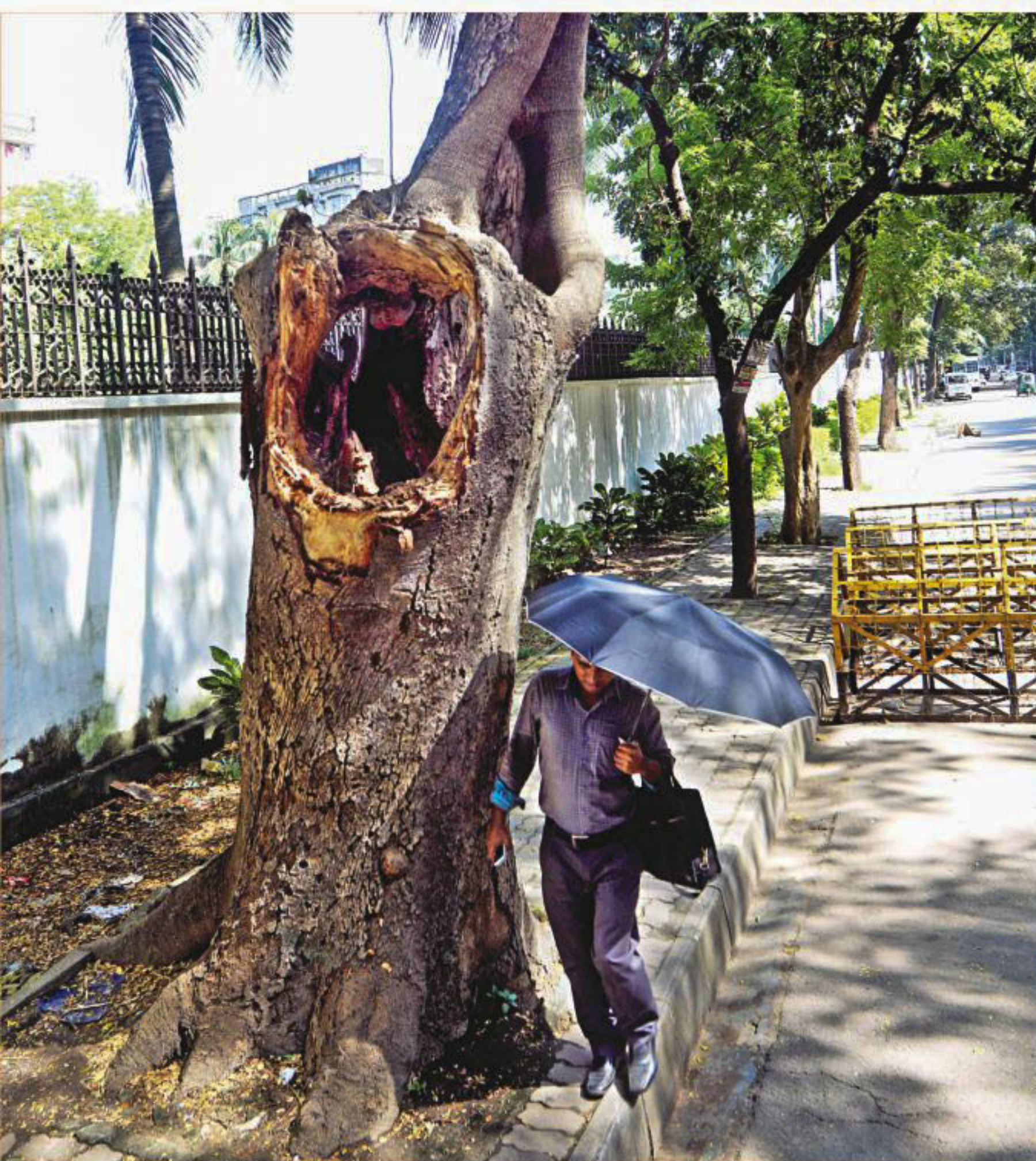
A large old tree with a hollow core puts passers-by at risk as its branches may break off at any moment. The photo was taken in the capital's Eskaton Garden recently.
