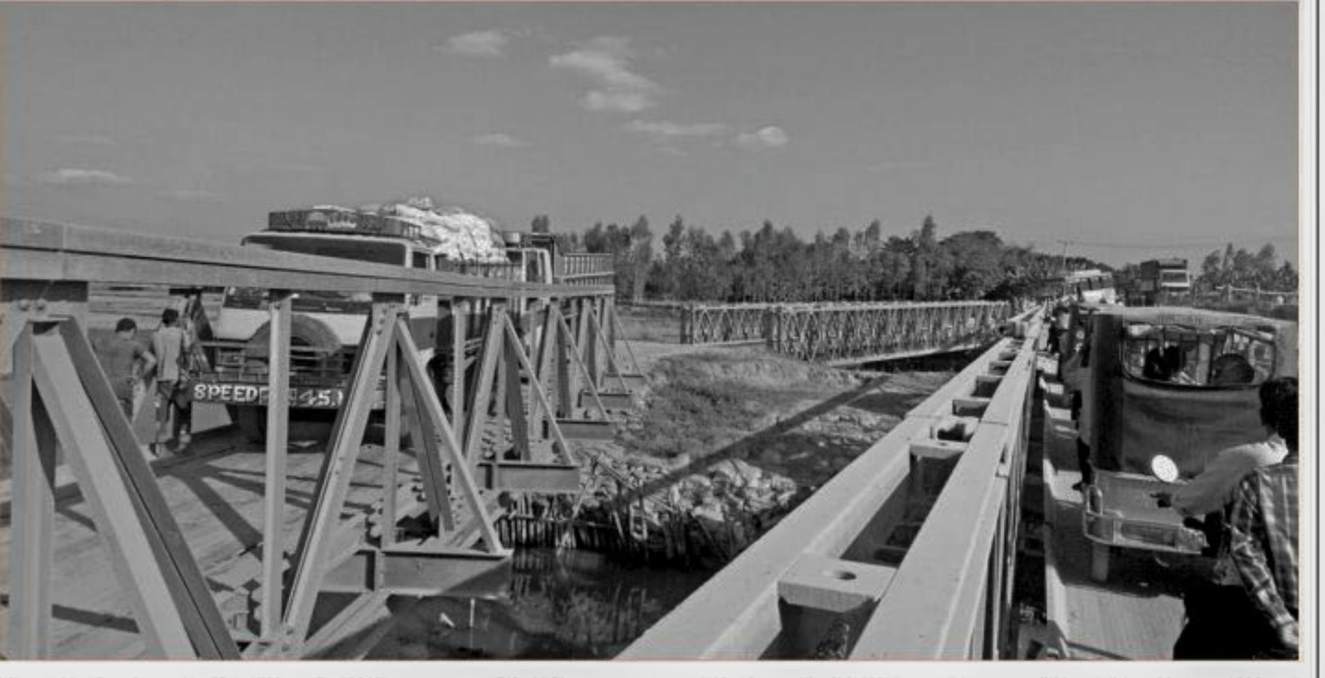
Steel deck of a Bailey bridge over the Swarnamoti river in Aditdari upazila of Lalmonirhat depressed when an overloaded truck with stones was crossing it on Sunday. PHOTO: STAR
