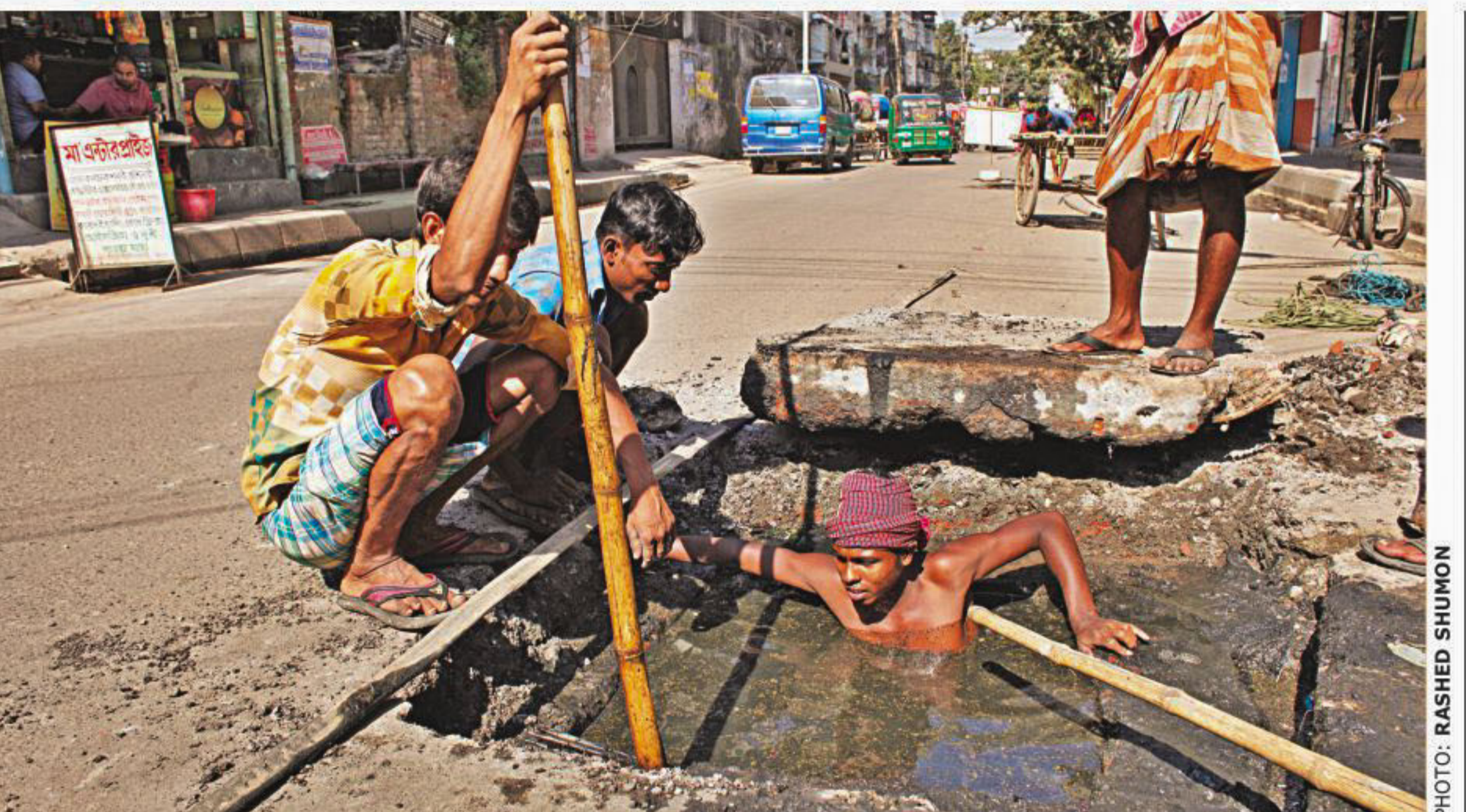
Oblivious of the dangers involved, workers of Dhaka North City Corporation get on with another day's work, getting down inside a sewer to clear it of a clog using their bare hands and feet and pieces of bamboo at Mohammadpur Madrasa Road in the capital. The photo was taken on Monday around 11:00am. PHOTO: RASHED SHUMON
