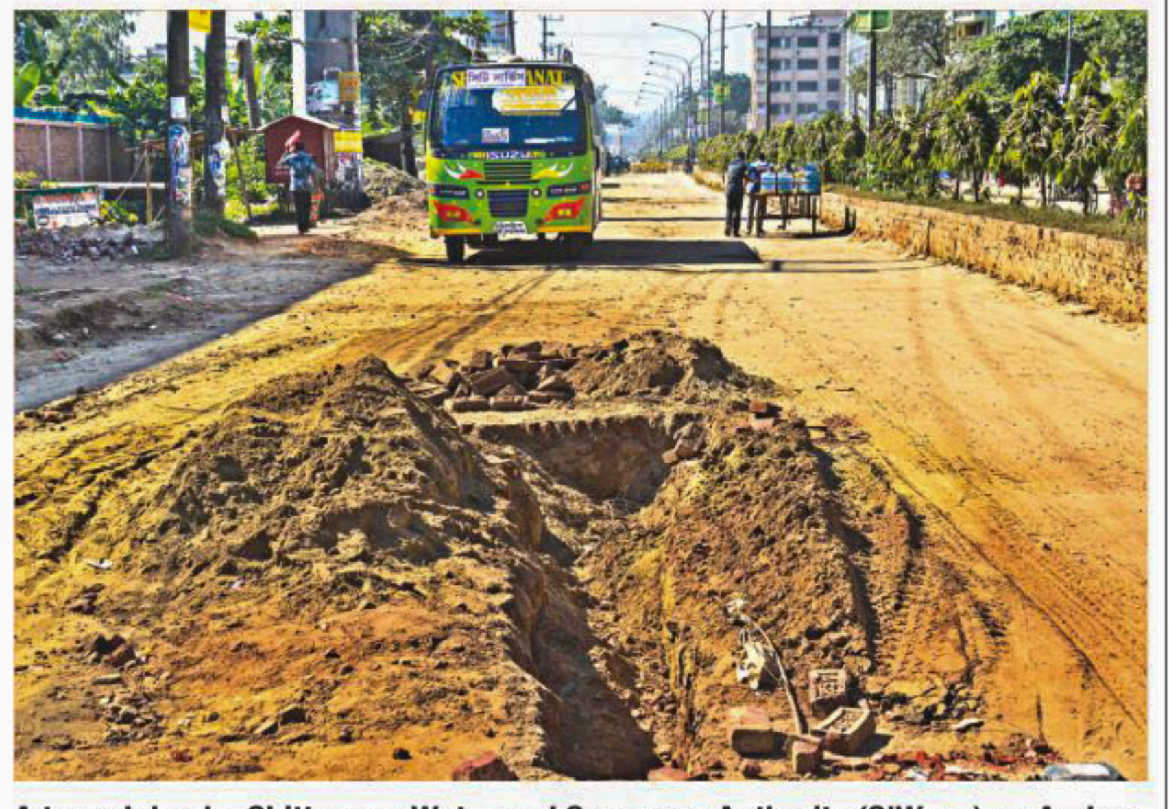
A tunnel dug by Chittagong Water and Sewerage Authority (C'Wasa) on Arakan Road in the port city for installation of water supply lines. The Bahaddarhat to Kalurghat section of the road, which was renovated at the end of 2013, has been again in a shabby condition, with the development work of Wasa adding to the woes. The photo was taken recently.
