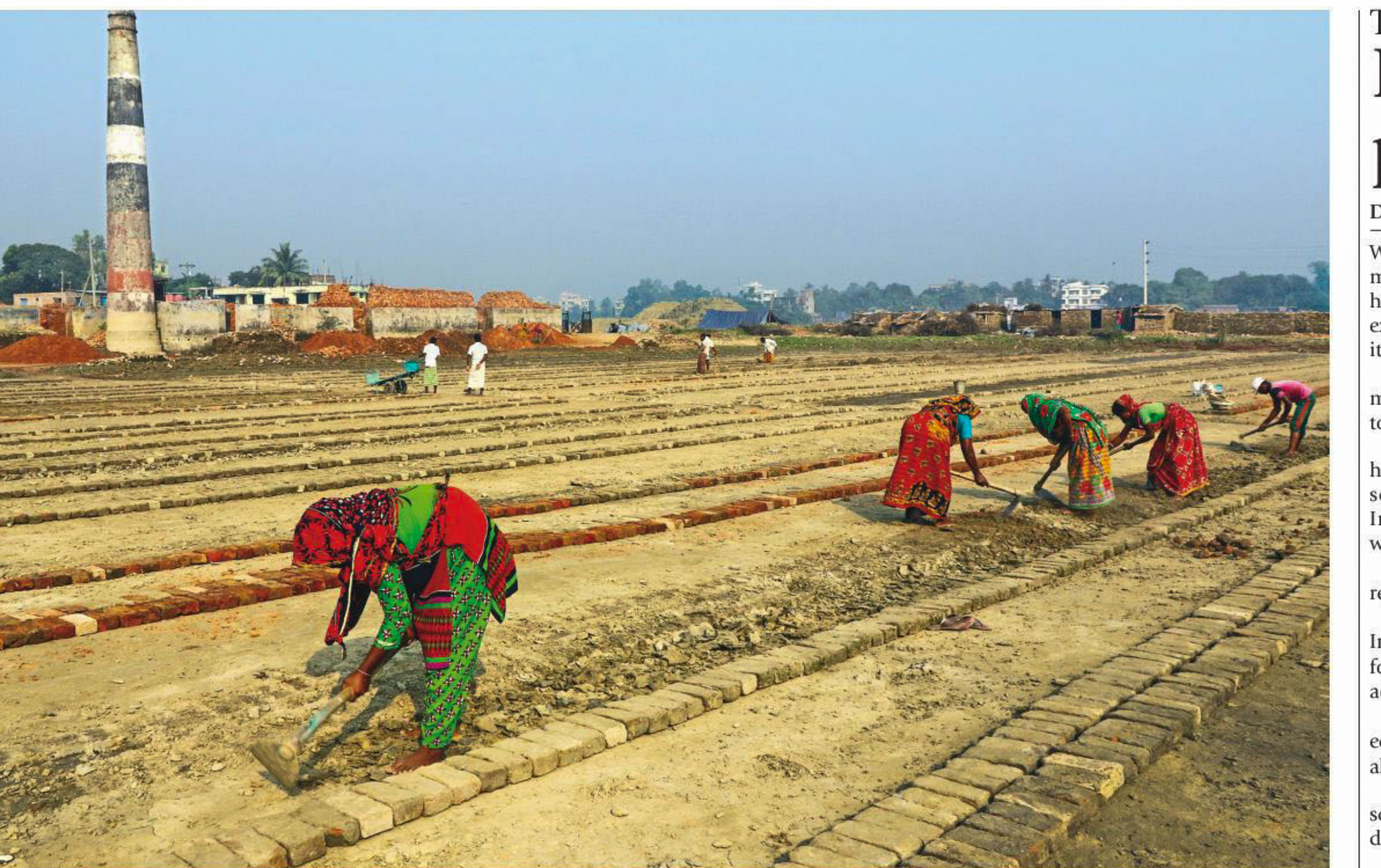
Though mainly female workers take up the role of preparing brickfields following the shutdown in production during the monsoon, they get Tk 350 toiling all day long, Tk 50 less than what males get, a disparity hirers justify claiming the latter "do more". The photo was taken at Savar's Boliarpur yesterday.
